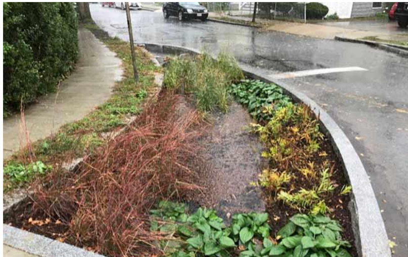
Green Infrastructure: Bioretention Basin construction at Egerton Rd/Herbert Rd, Arlington, September 2018. Two similar rain gardens will be constructed in East Arlington in 2020.
