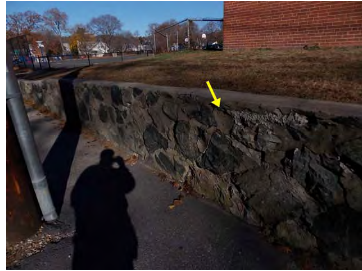
This retaining wall (adjacent to Pleasant Street) has sections of mortar loss
