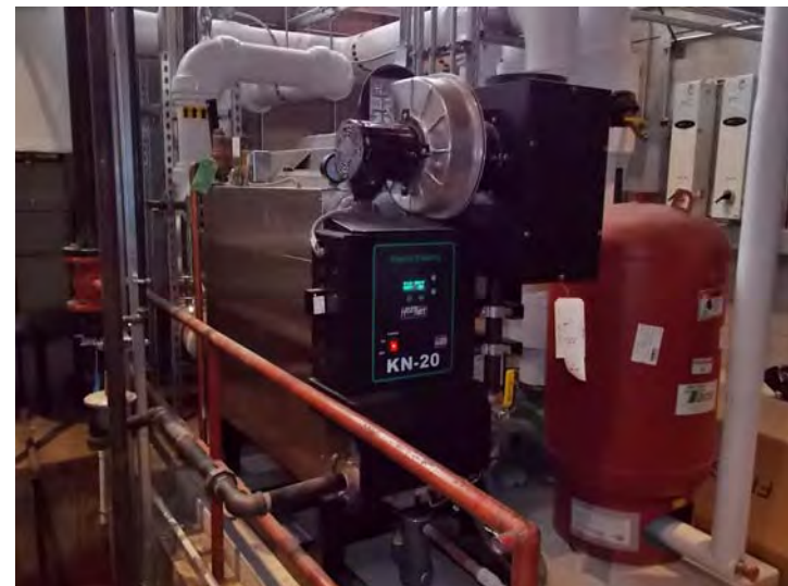
This natural gas-fired condensing boiler produces hydronic heat for the new wing.
