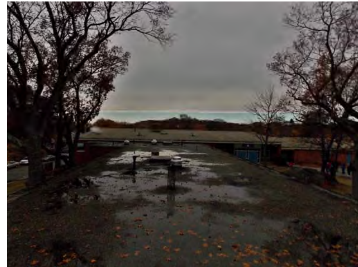
The original building has an older tar and gravel roof covering (over both the flat and pitch sections). Despite the amount of standing water (ponding) no active leaks were reported.
