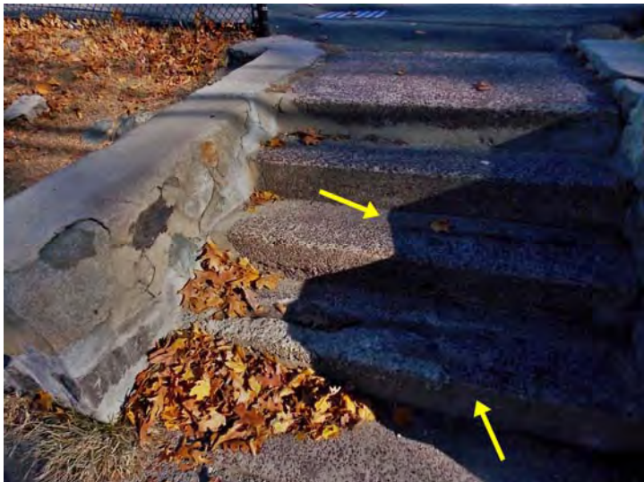
These concrete steps (near the main gym) have spalled treads.
