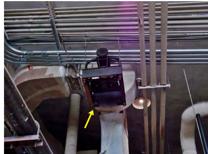
An induced draft fans on one of steam boilers, to assist in venting of flue gases.
