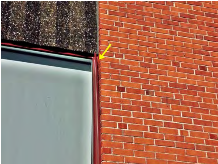
A portion of the metal trim at this window has come loose.
