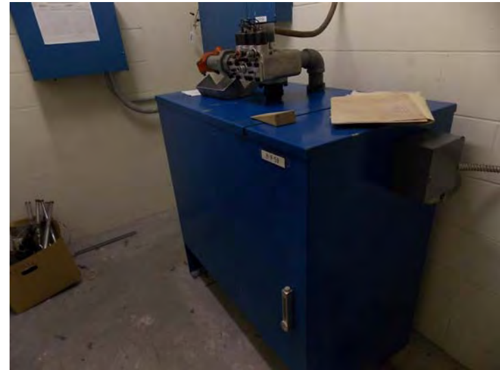
This is the elevator's hydraulic pump station.
