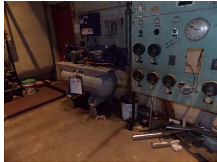
This original pneumatic (compressed air) system is used to control thermostats and motorized valves throughout the original building.
