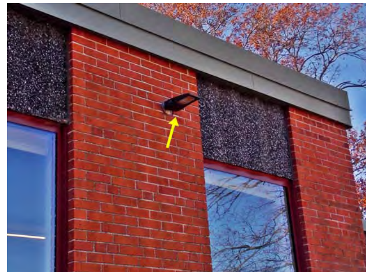
This is LED light fixture should provide a long-lasting and energy efficient lighting source.
