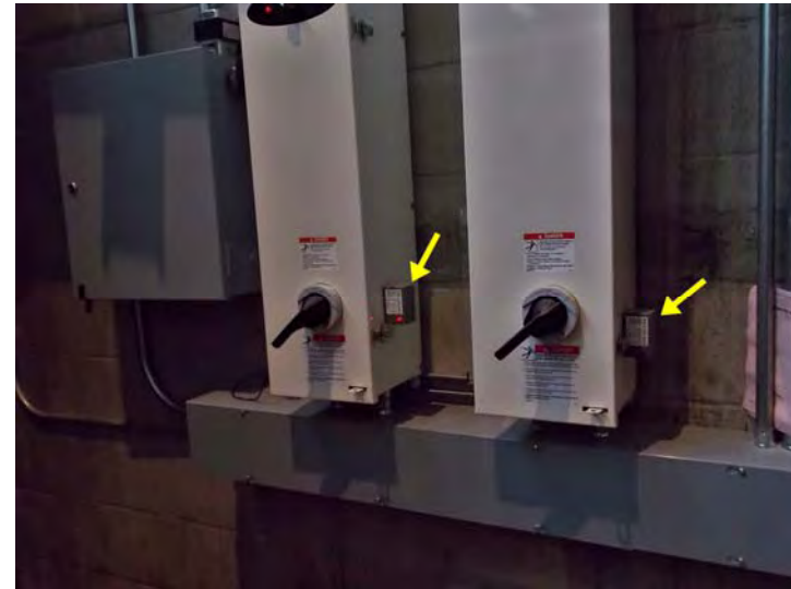
These are the variable frequency drives (VFDs) that control the hydronic pumps. Note the communication modules (arrows) that enable the school's energy management system to control the VFDs remotely.
