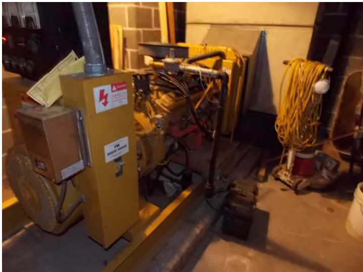
Emergency power is provided by this natural gas powered generator (49 kW).
