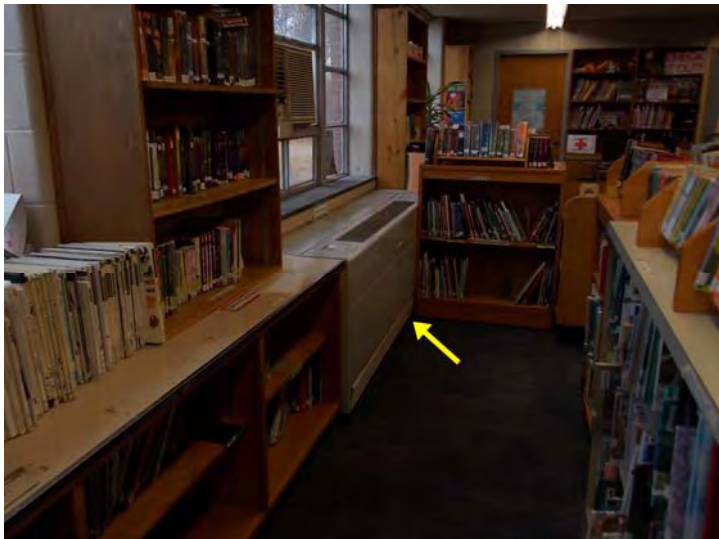
One of the steam-heated through-wall convectors.
