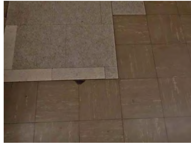
A repaired flooring section in a classroom in the wing. The lighter colored tiles are vinyl composite tiles (VCT) used to replace damaged sections of the original smaller vinyl asbestos tiles (VAT).
