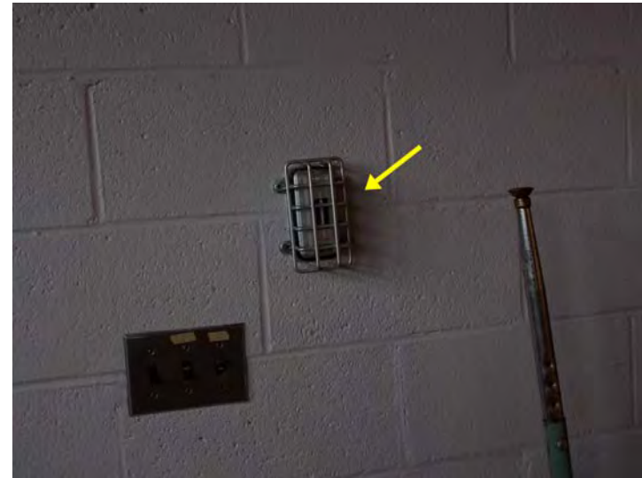
One of the pneumatically-controlled thermostats.
