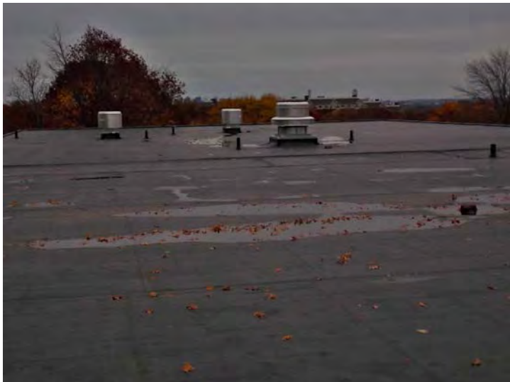
The new wing has a rubber membrane roof covering and internal drains.
