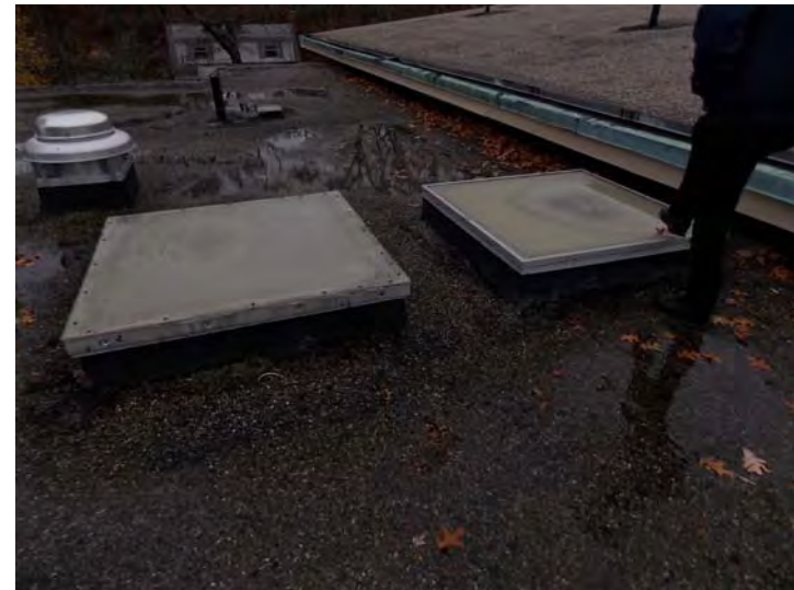
A pair of skylights over the administration section of the original building.
