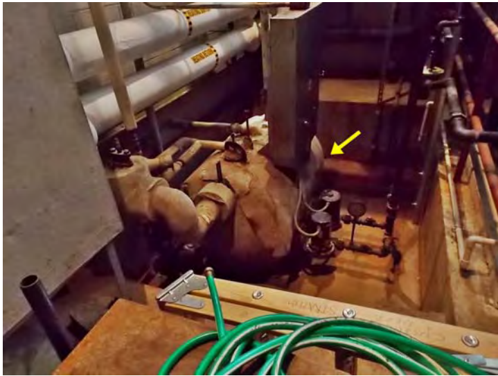
This is the main condensate receiver; condensed (cooled steam is collected in this vessel for re-use).
