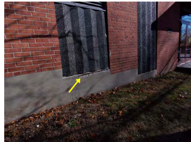
This concrete wall section has spalled and exposed the steel reinforcement (rebar) at this window assembly.
