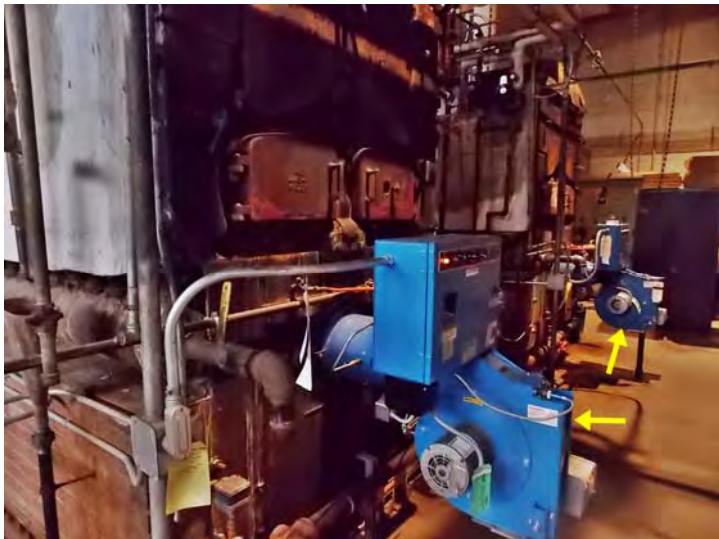
This pair of original natural gas-fired low pressure steam boilers serves the original building. The boilers have been upgraded with new forced draft burners.
