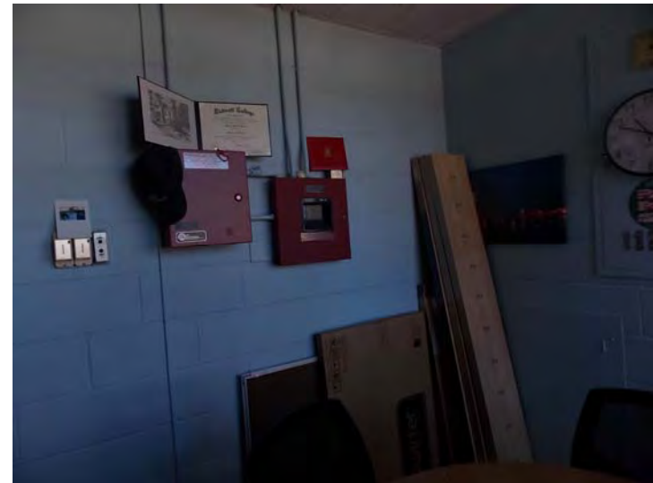
A view of the main fire alarm control panel.
