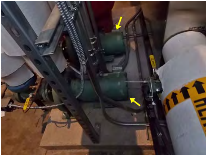
These are the variable speed 5 hp pumps used in a lead/standby manner to distribute hydronic heat throughout the new wing.
