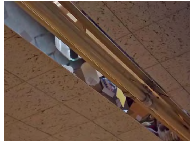
This is typical most of the lighting fixtures throughout the school: high efficient fluorescent lamps (T8s with electronic ballasts). Fixtures have a reflector surface to improve light output.
