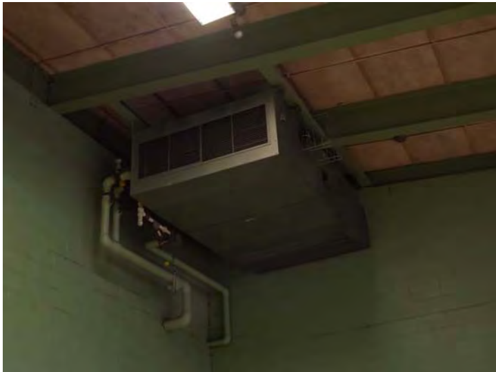
An air handler in the main gym; this unit has a steam coil to provide warm air.
