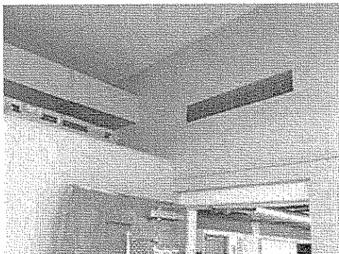
Ventilation Register in Office (typ.)
