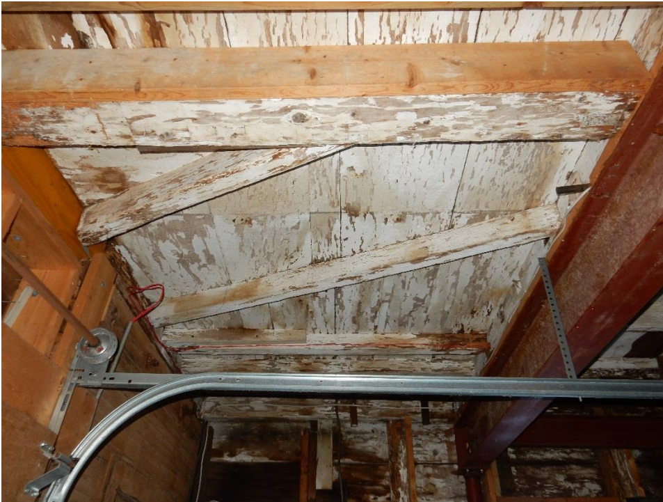
20. Mislocated second floor wood joists which appear to have been moved when installing steel shores now not adequately supporting board flooring.
