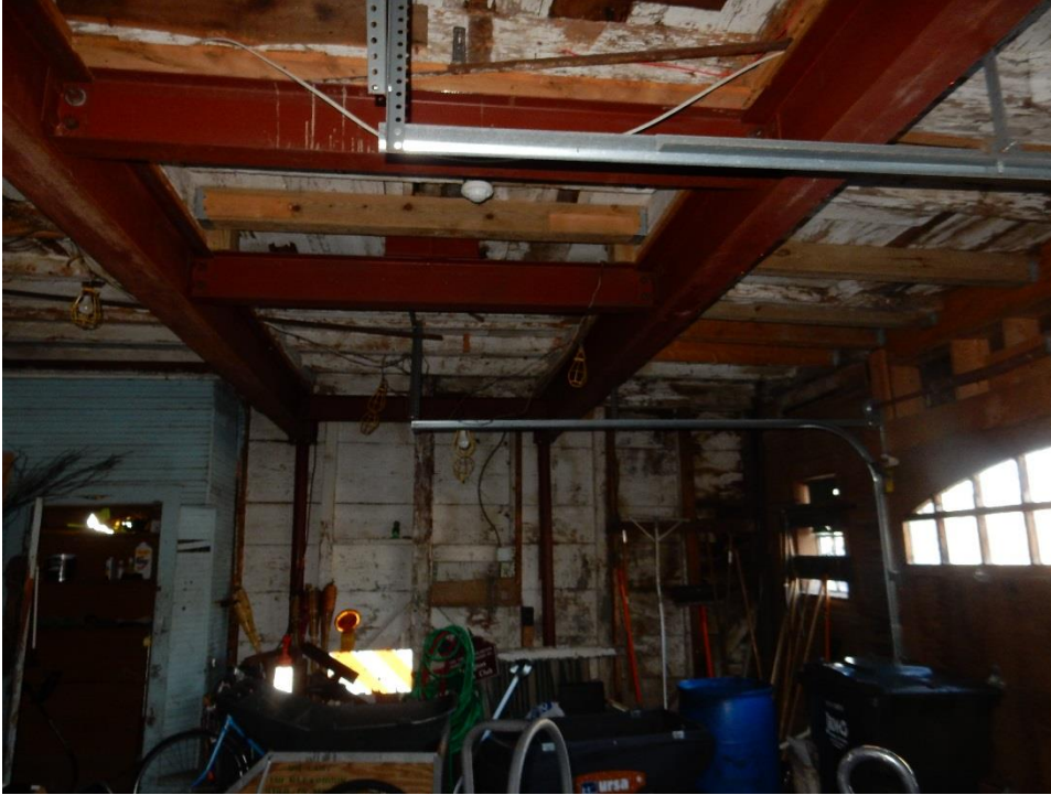
17. Underside of second floor framing in two-story building. Steel beams supported on pipe columns which shore second floor. Existing wood beams are piggybacked on top of the steel beams.
