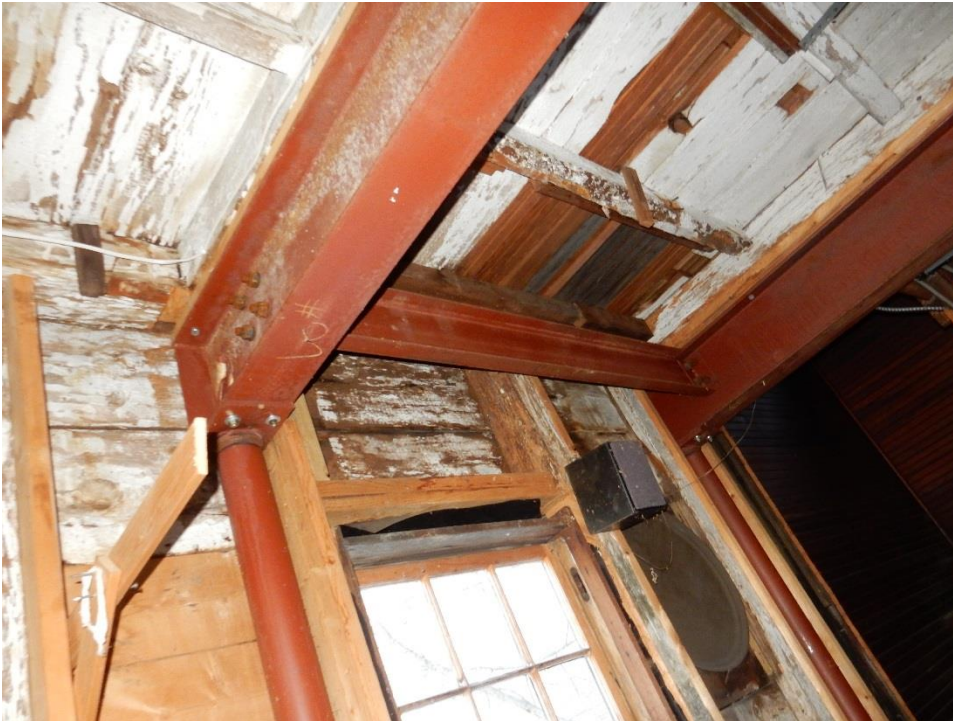
18. Underside of second floor framing in two-story building. Steel beams are supported on pipe columns next to stairs.
