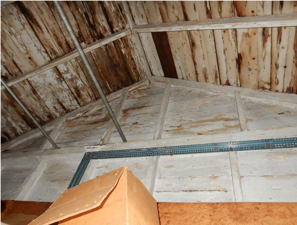
16. Gable wall and roof framing over aforementioned bay. Rafters appear intact. Board sheathing is stained from past moisture.
