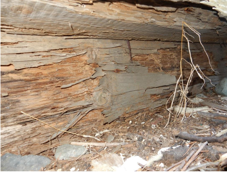
9. At south face of one-story area, cinder block foundation which caps rubble foundation and supports wood sill is missing. The vertical board appears to be the backside of a nailer that supports interior board finishes.
