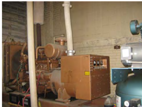
Building D's gas fired generator.
