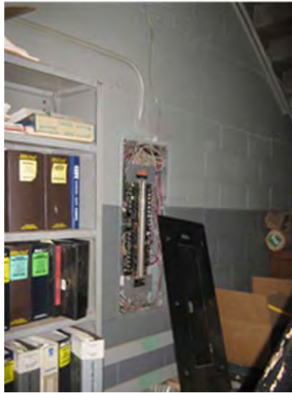
Building D electrical panel under first floor central stairs.
