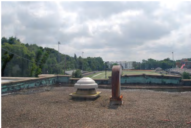
Ponding water on the old roof.
