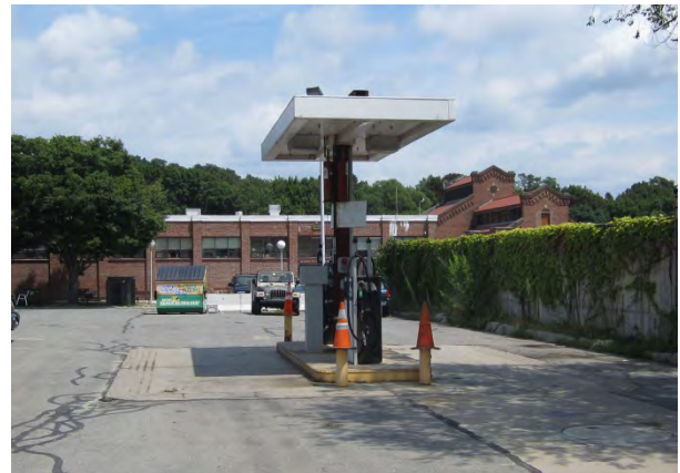
Small canopy provides inadequate weather protection.
