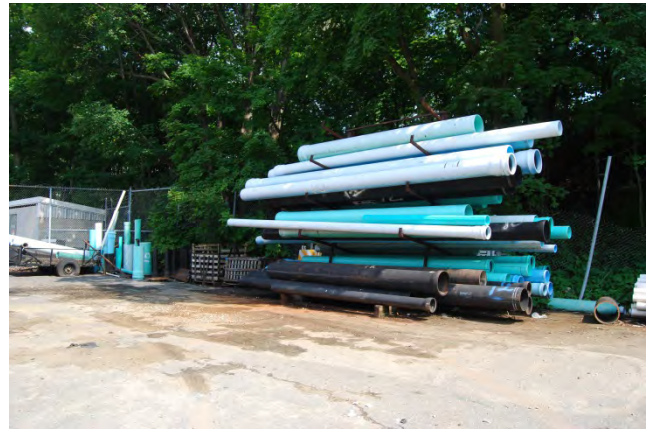
Supplies left exposed to the weather rapidly deteriorate.
