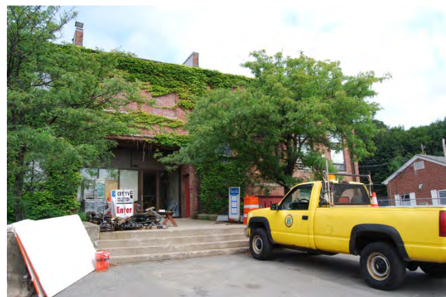
Aggressive plant materials on rear facade.
