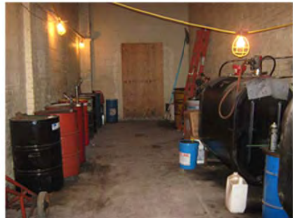
Oil/hazardous material storage lacks an exhaust system or explosion-proof fixtures.
