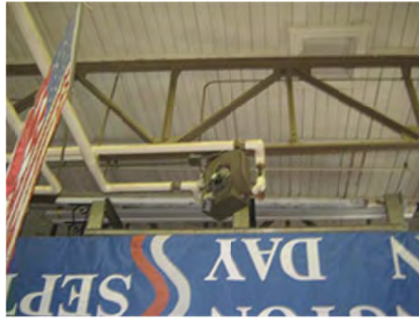
Heaters located in the Sign Shop of Building A
