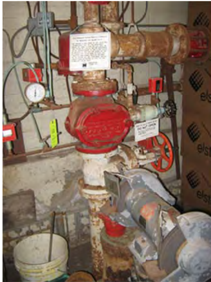
Building D's sprinkler system is in need of updating.
