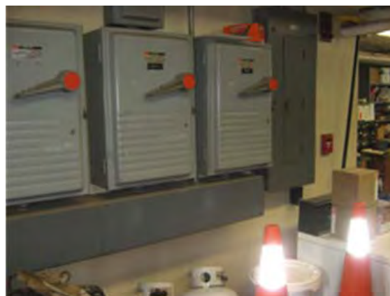
Building A electrical panels in entrance of Sewer Shop.
