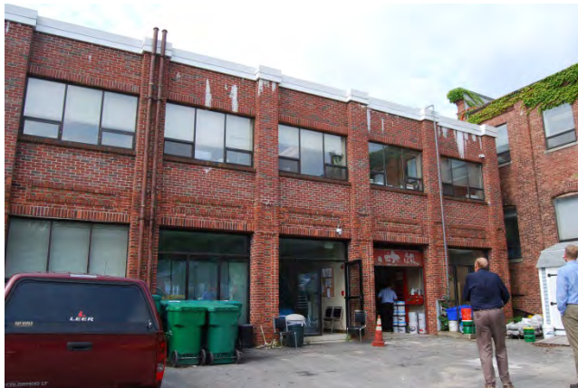
Leaching bricks on the rear of the building.
