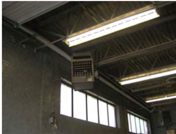
Local heating units mounted in Building D.
