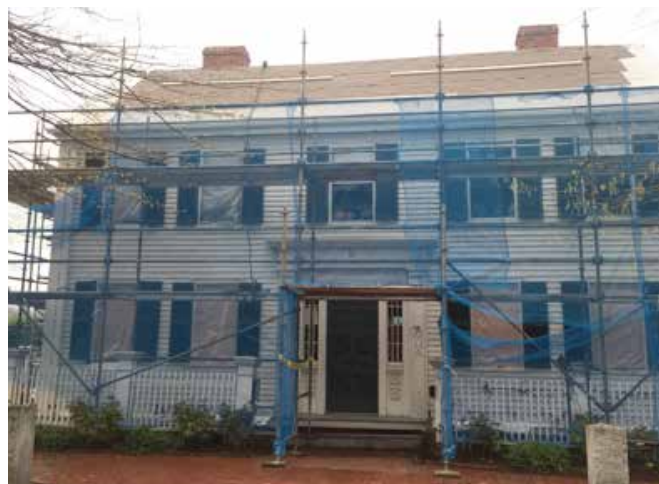
Jefferson Cutter House in May 2016. Scaffolding was erected as part of a full exterior restoration of the building including new roof, refurbished windows, shutters, doors, and repairs to rotted exterior clapboards and trim. Photo courtesy of Sarah Burks.
