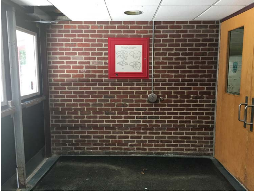
3. Existing Entry Vestibule wall. Existing fire annunciation panel to remain and be protected during construction. New transaction window shall be installed on left of fire annunciation panel shown above.
