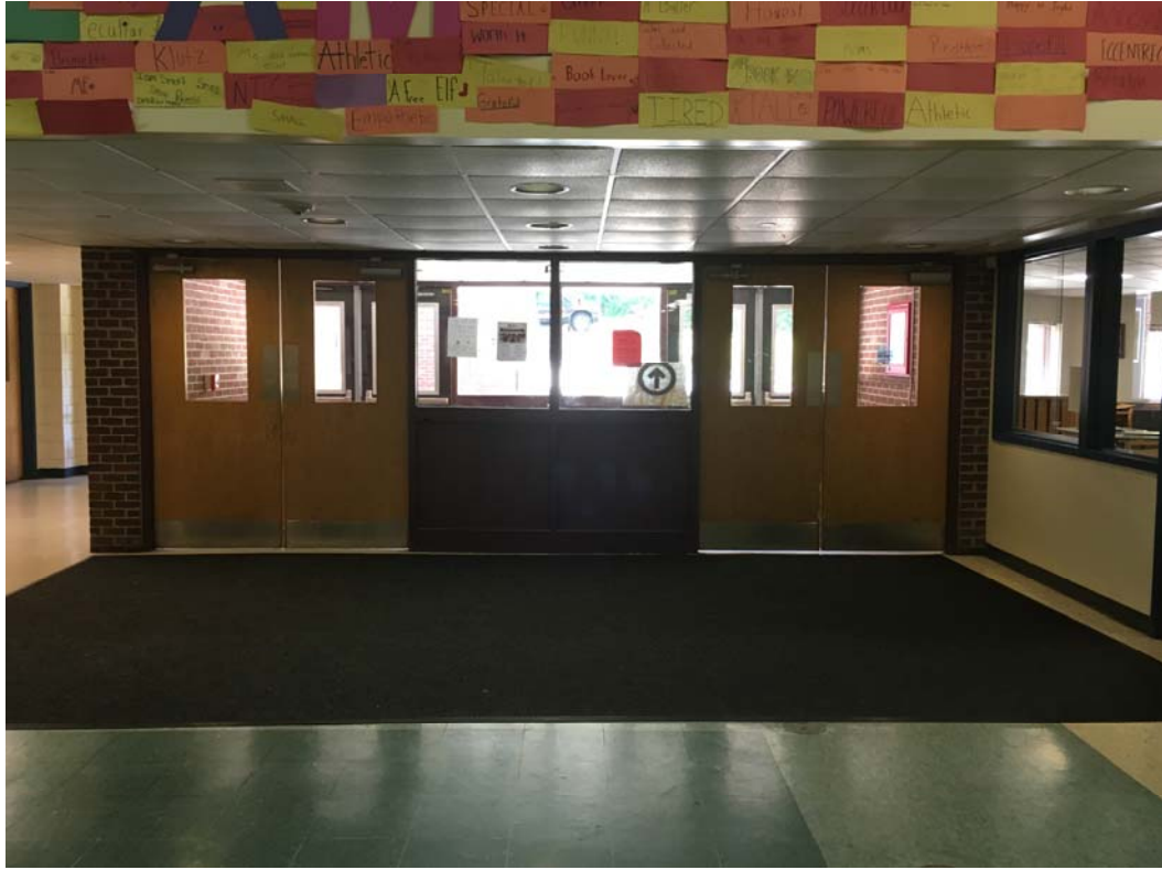
1. View of existing interior vestibule doors. Door shown on right shall be replaced with new pair of doors and hardware as sown on drawings.
