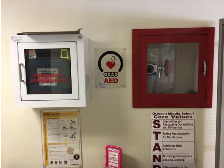
7. Existing AED cabinet and fire valve cabinet. Relocate AED cabinet as required for installation of new wall.
