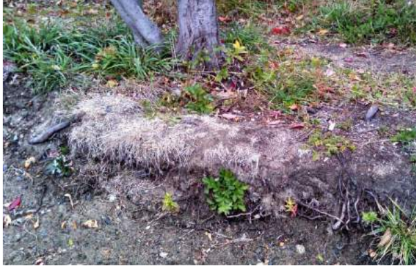
Photograph 9: Eroded Pond Edge
