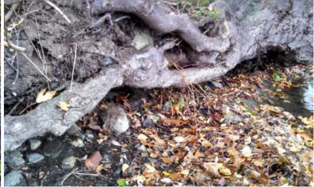
Photograph 10: Exposed Tree Roots Being Undercut
