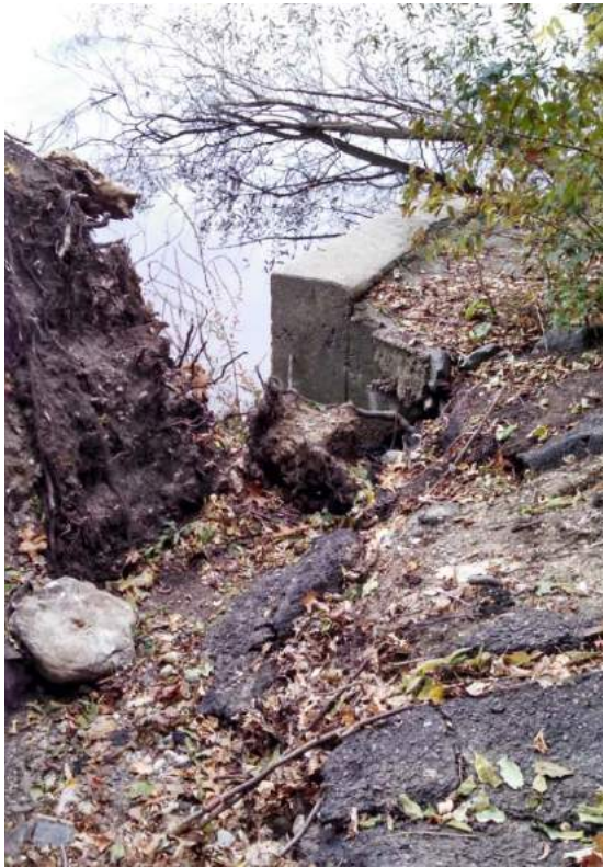
Photograph 16: Eroded Slope near Stormwater Outfall
