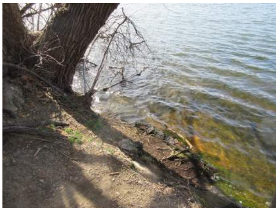
Photograph 3: Erosion and Lack of Vegetation
