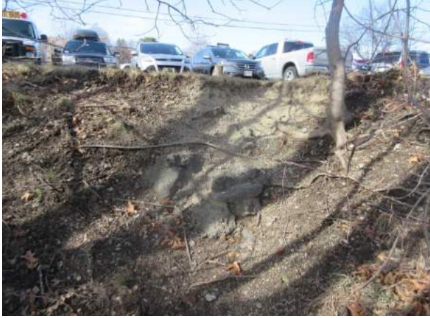
Photograph 11: Steep Eroded Slope
