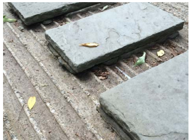
Failing Mortar Stepping Stones
