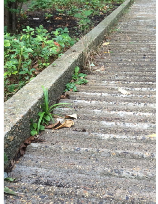
Weeds Growing in Spillway Joint
