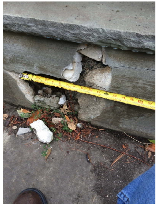
Close up on Failing Wall
