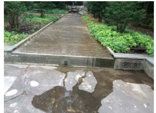
Unlevel Spillway in Operation
