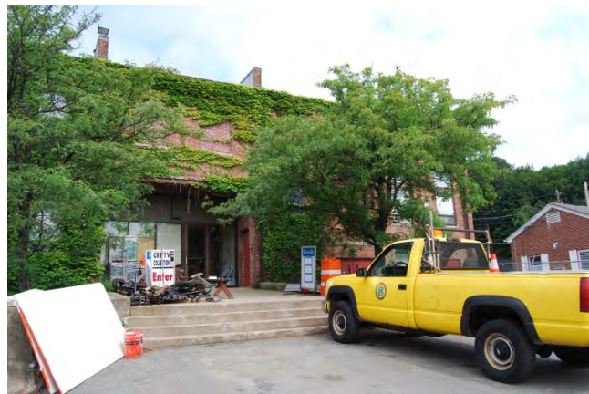
Aggressive plant materials on rear facade.
