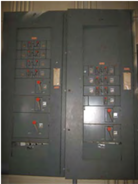
Electrical panels located in Building B.
