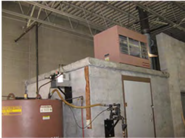
Waste Oil Heater in Building C
