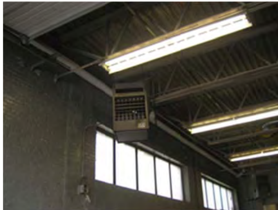
Local heating units mounted in Building D.
