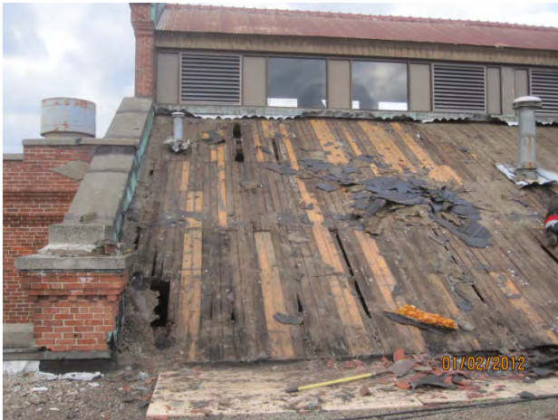
Split and cracked boards under the historic tile roof.
