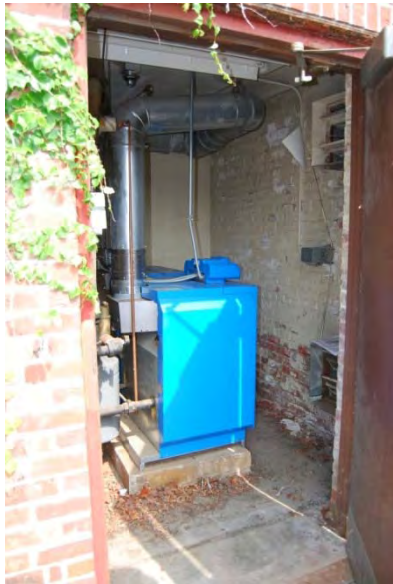
Building A's boilers
