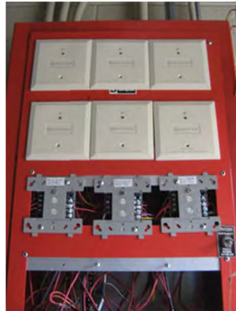
Fire Alarm panels located in Building B.
