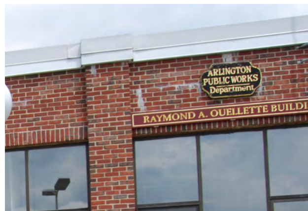
Leaching on the front of the building.
