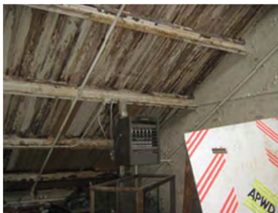
Unit heater on level two of Building D.
