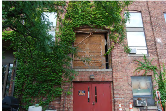
Deteriorated wood sign shop door still in use.
