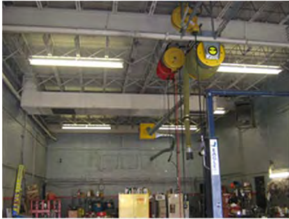
Vehicle Exhaust and Ductwork
