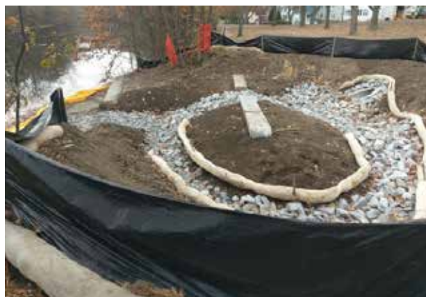
New stormwater infrastructure along the Mystic River.
