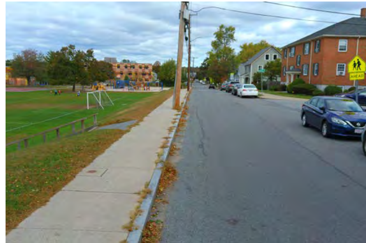
Figure 62. Lussiano Field sinks below curb along N Union St.
