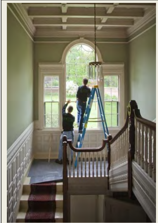
Lyman Estate weatherization improvements by Historic New England included wood window rehabilitation.
