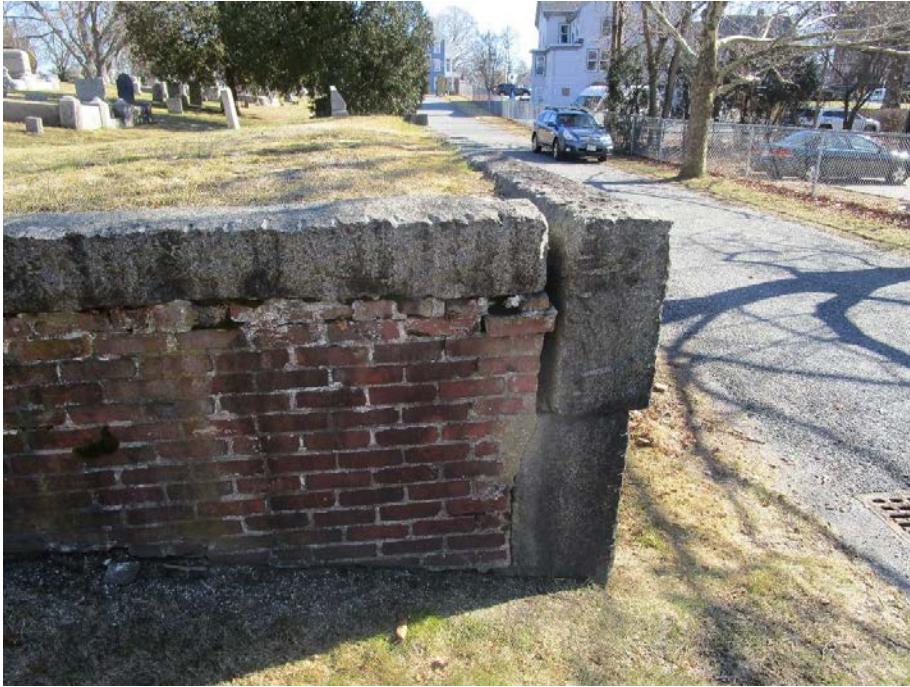
The brick retaining wall is leaning outward and the upper courses are debonded.
