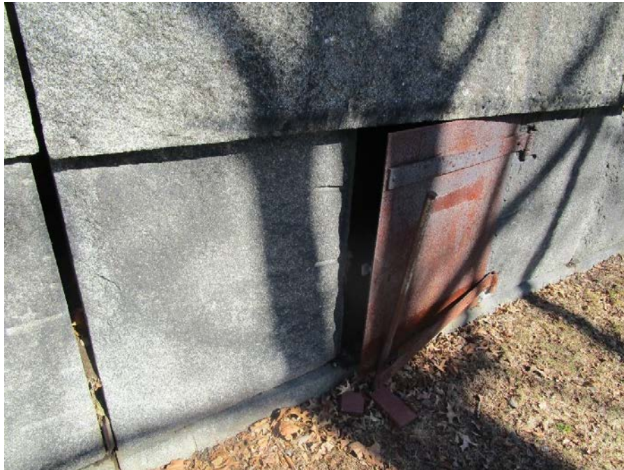
The metal doors are badly corroded and the straps securing them to the hinges are either missing or detaching from the sheet metal. The door closure system – a bar hammered into the ground is not very secure.
