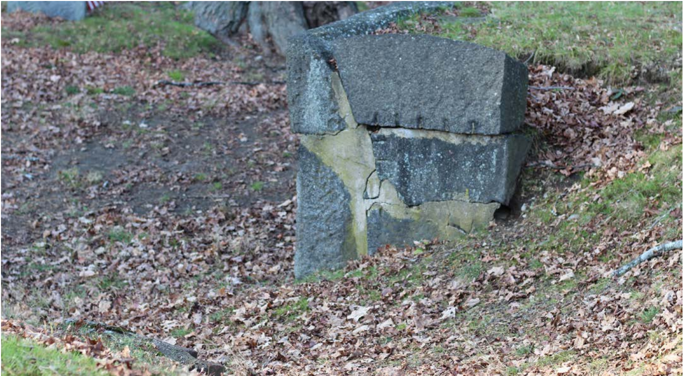
Masonry Side Walls of OBG Northeast Tombs Have Shifted
