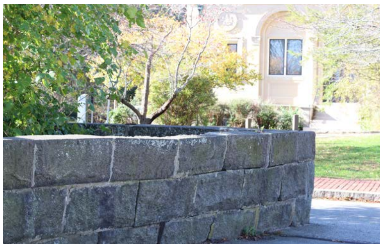
6. Northeast wall - stone, area of bulging
