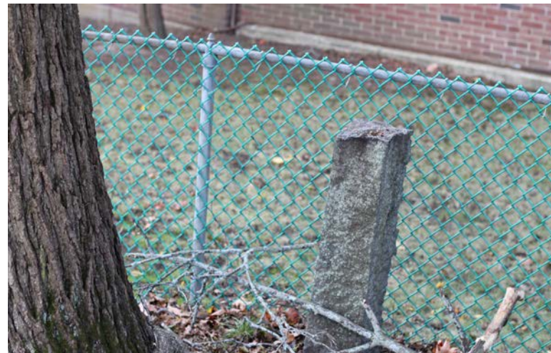
12. Granite posts, missing iron rail
