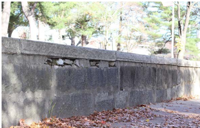
4. Pleasant Street wall - mortar missing from joints
