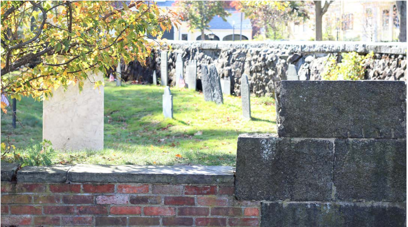
OBC Walls Vary in Their Construction and Condition; View of Brick, Granite Block and Fieldstone Walls Beyond
