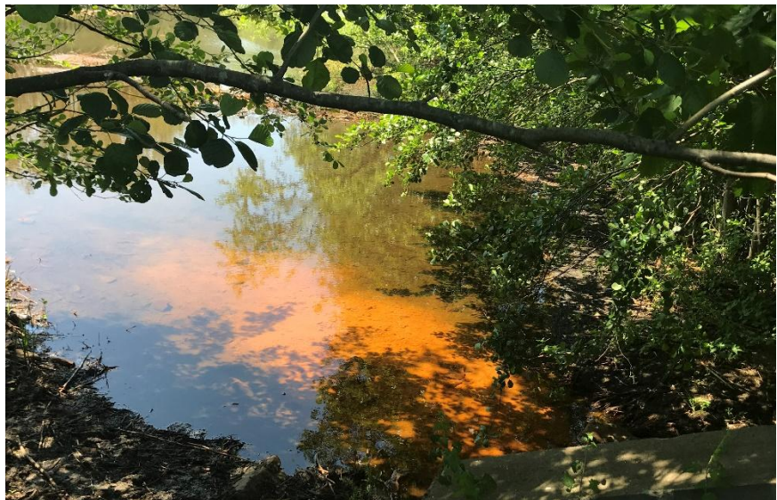
Reeds Brook culvert to detention pond showing iron flocculation, Spring 2018
