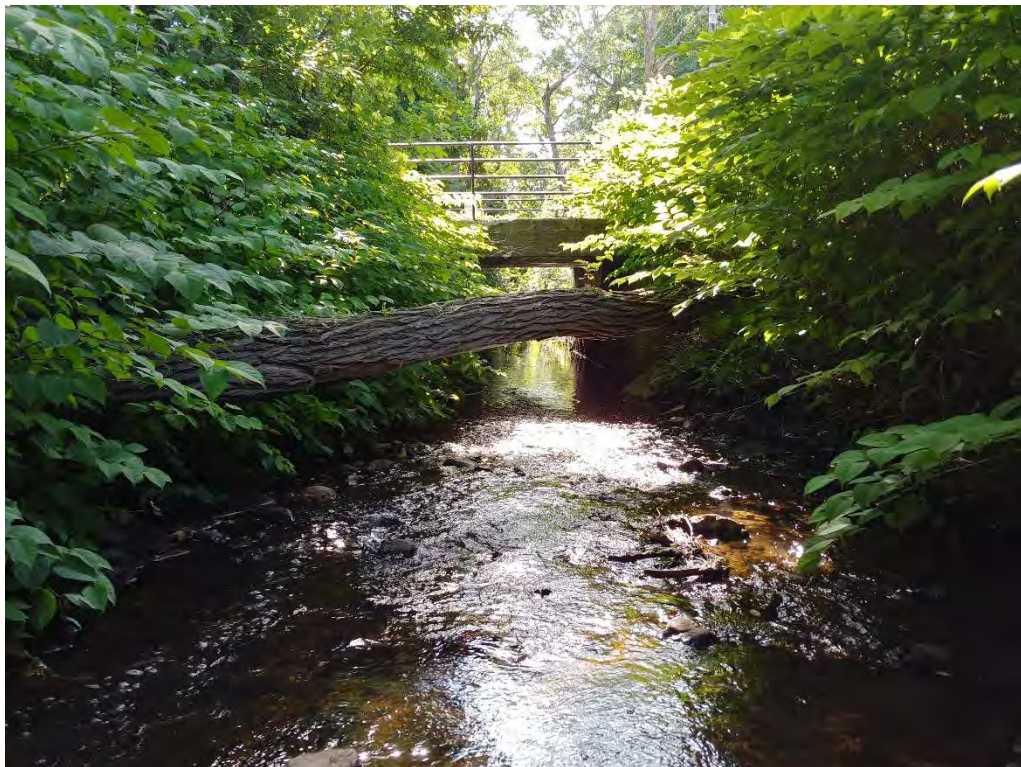
Photo 2. View of Bank Series AB between flags AB-3 and AB-103, looking east towards the concrete bridge connected to Mill Brook Drive.
