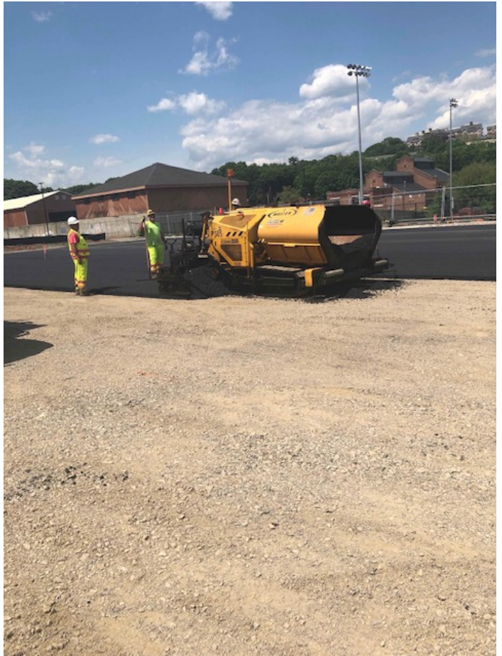
Photograph 3: Allied Paving making passes with the paver in the west parking lot (6/4/20)
