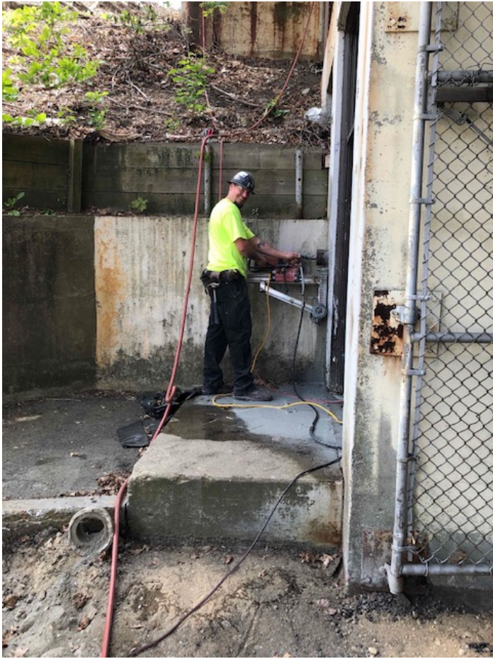
Photograph 5: Coring holes in the Auditorium building for installation of a new temporary fire protection line (6/3/20)
