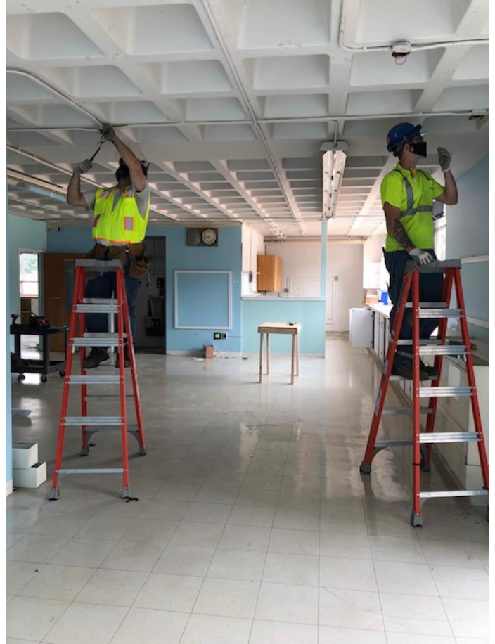
Photograph 2: Wayne J. Griffin electric beginning phase one demo in the Downs building (6/3/20)
