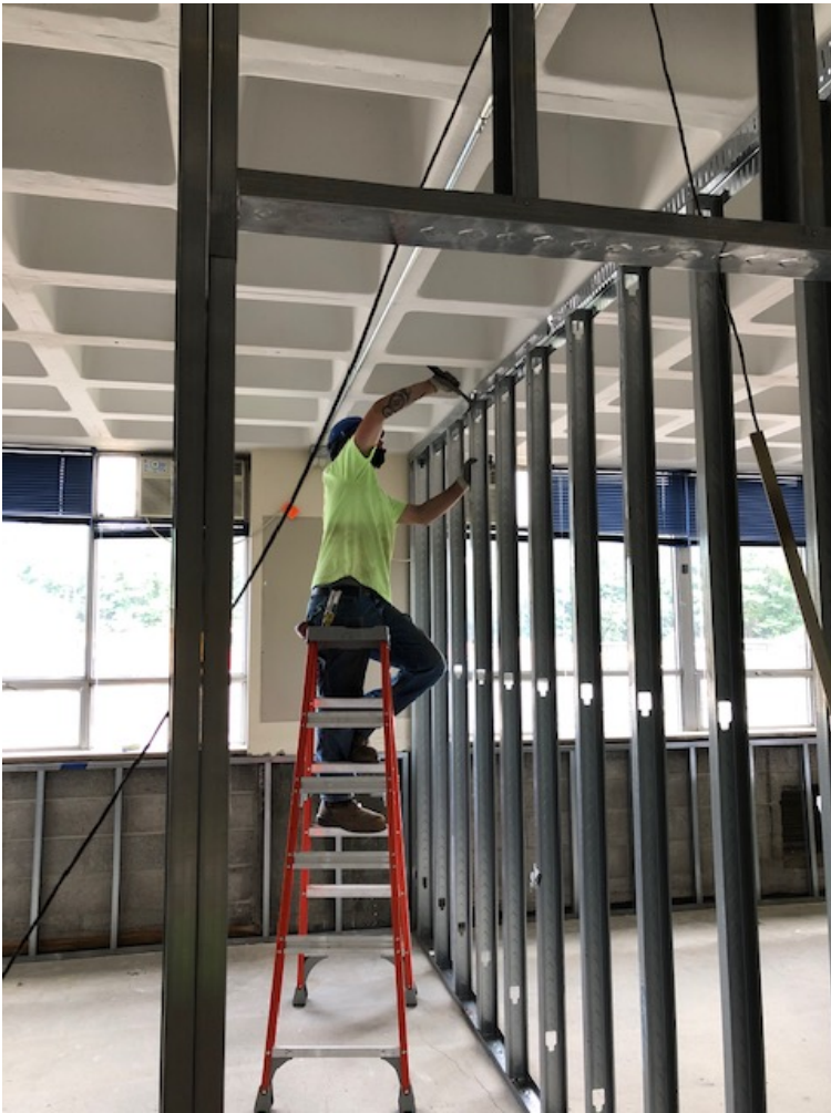
Photograph 3: Griffin laying out electrical service for new temporary guidance offices in Downs building (6/26/20)
