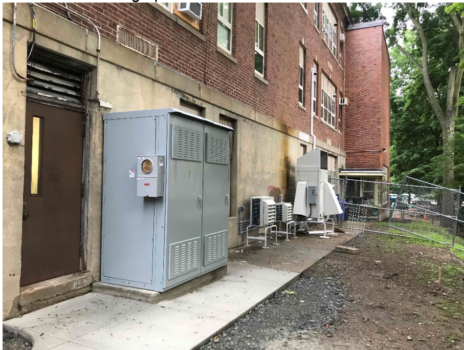
Photograph 8: Electrical switchgear and condenser units installed
