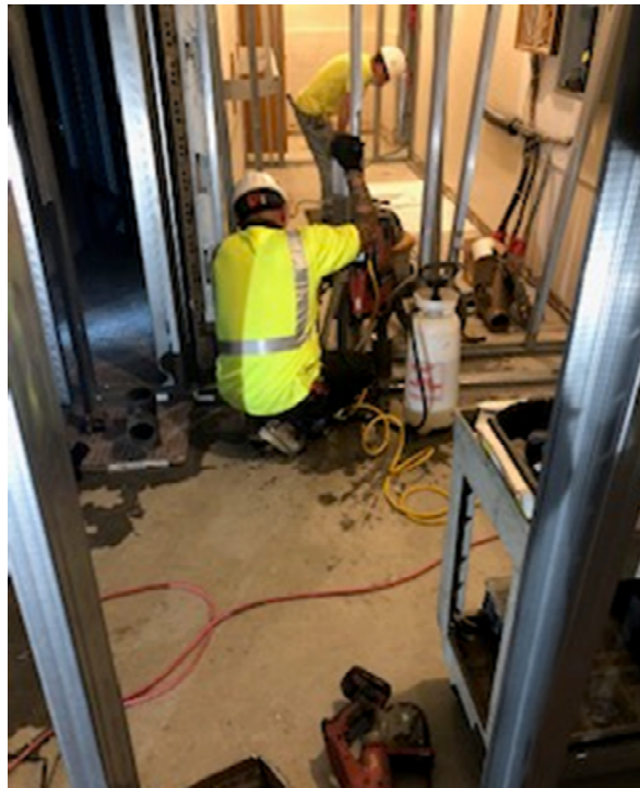
Photograph 6: Irvine bringing in plumbing for new bathroom in the new swing space at Downs Building
