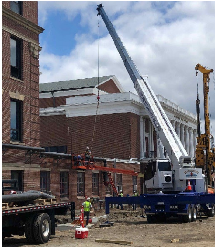
Photograph 4: PJ Kennedy Securing Gas Pipe as seen from Mass Ave Front Lawn
