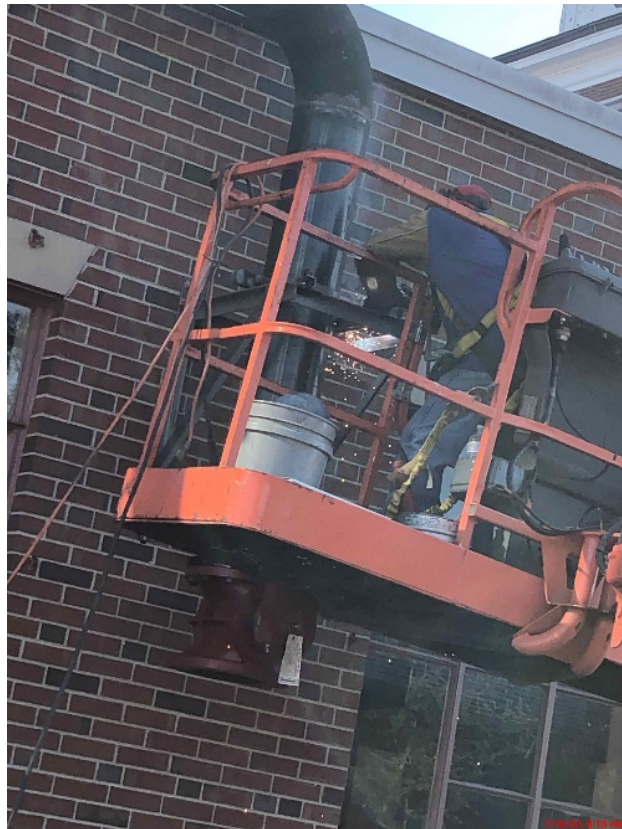
Photograph 2: PJ Kennedy Welding Gas Pipe as seen from Mass Ave Front Lawn
