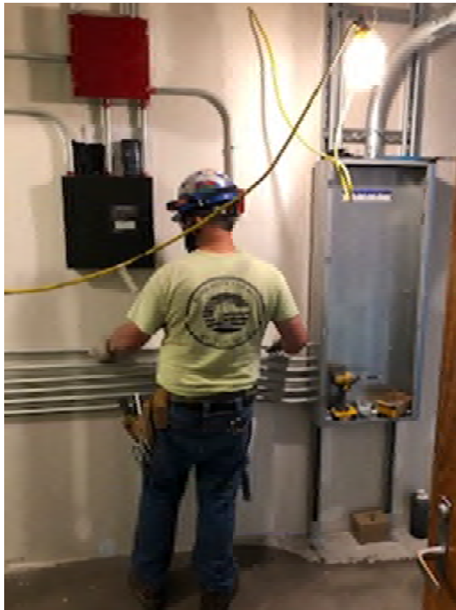
Photograph 4: Griffin Piping in new panel in Downs building
