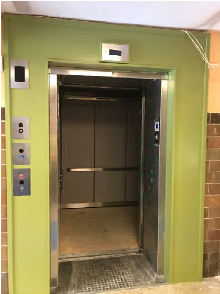
Photograph 7: Elevator cab and finishes on 1 st floor
