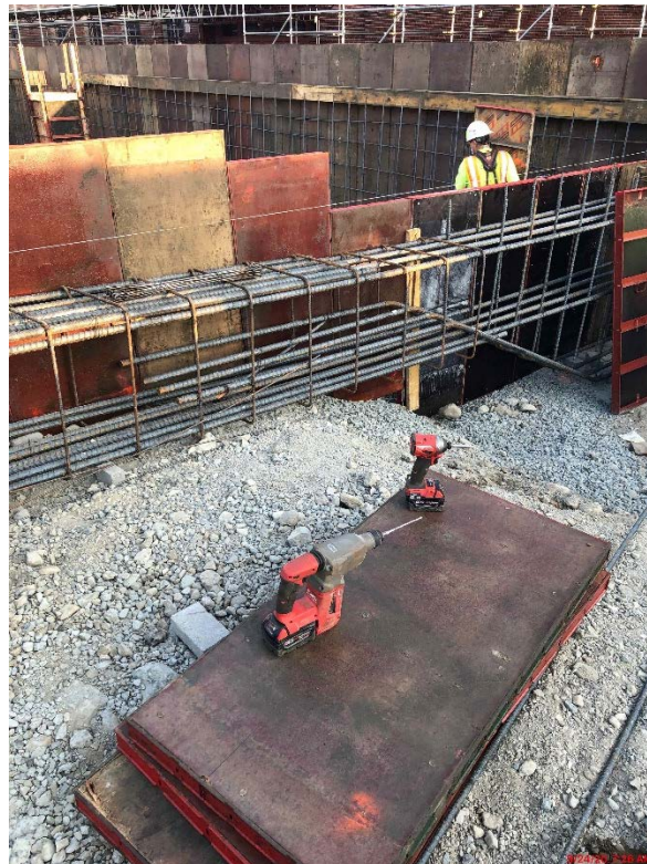
Photograph 4: Re-bar tied for continuous footing along the eastern wall for Phase 1 new building foundation
