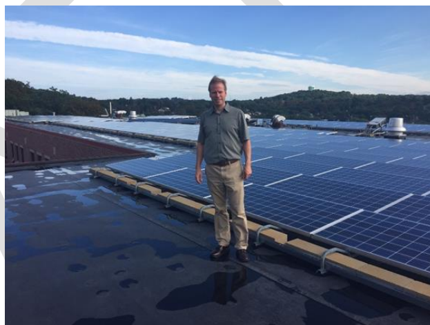
Solar array, Ottoson Middle School
