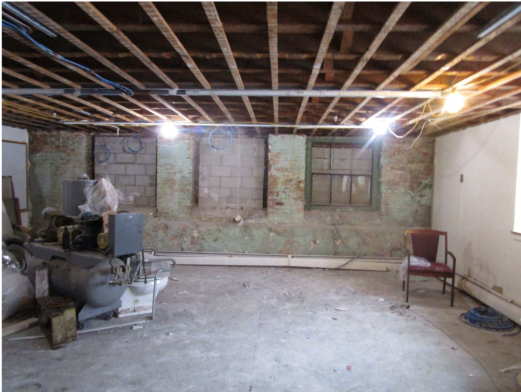
East wall of Yoga room on GF. Old windows previously blocked in due to raising of exterior grade
