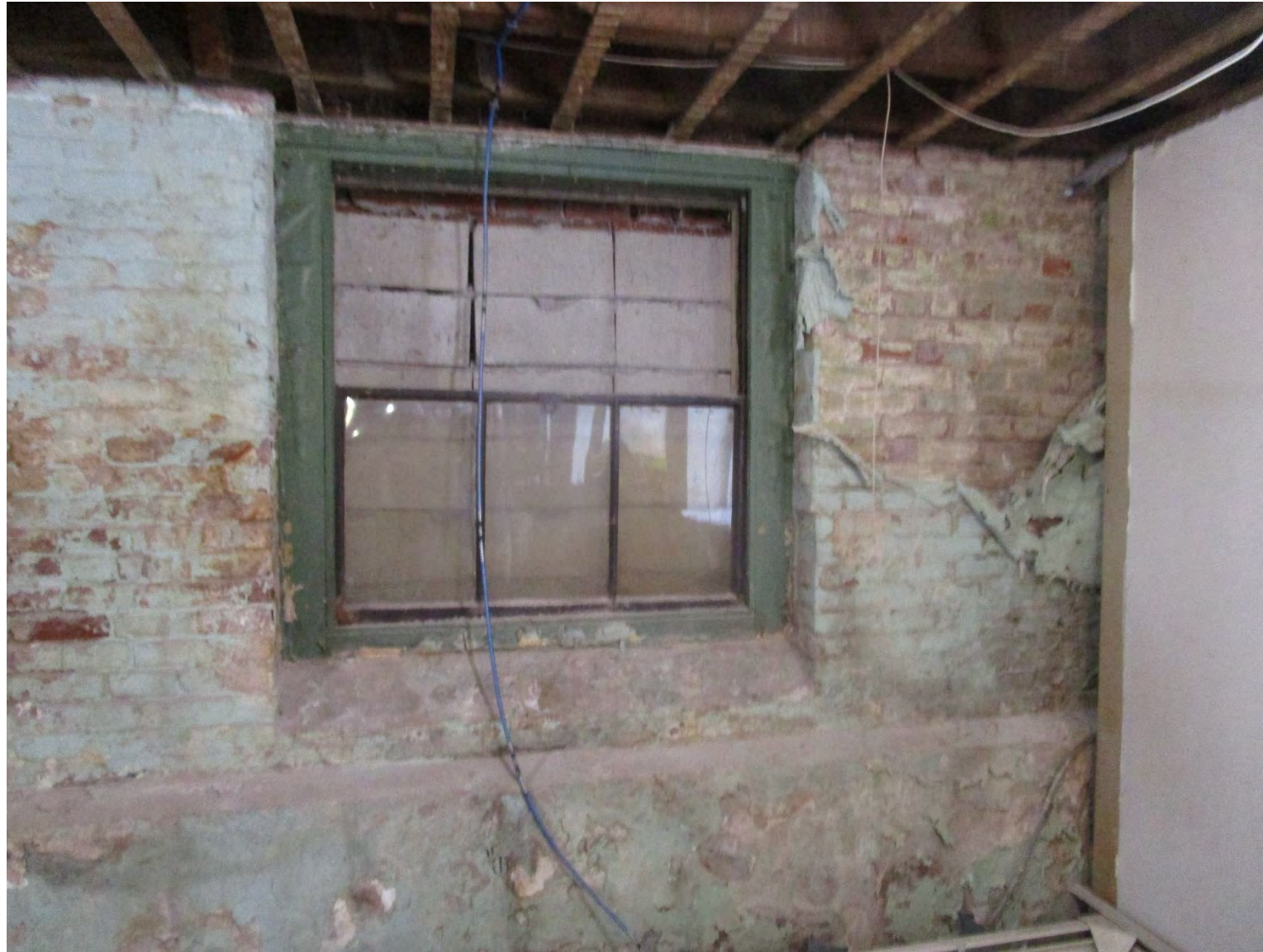
Previous contractor failed to fully remove one window frame and sash before blocking in the opening and installing drywall on interior. Moisture infiltration evident. Mitigated by new work on east side.
