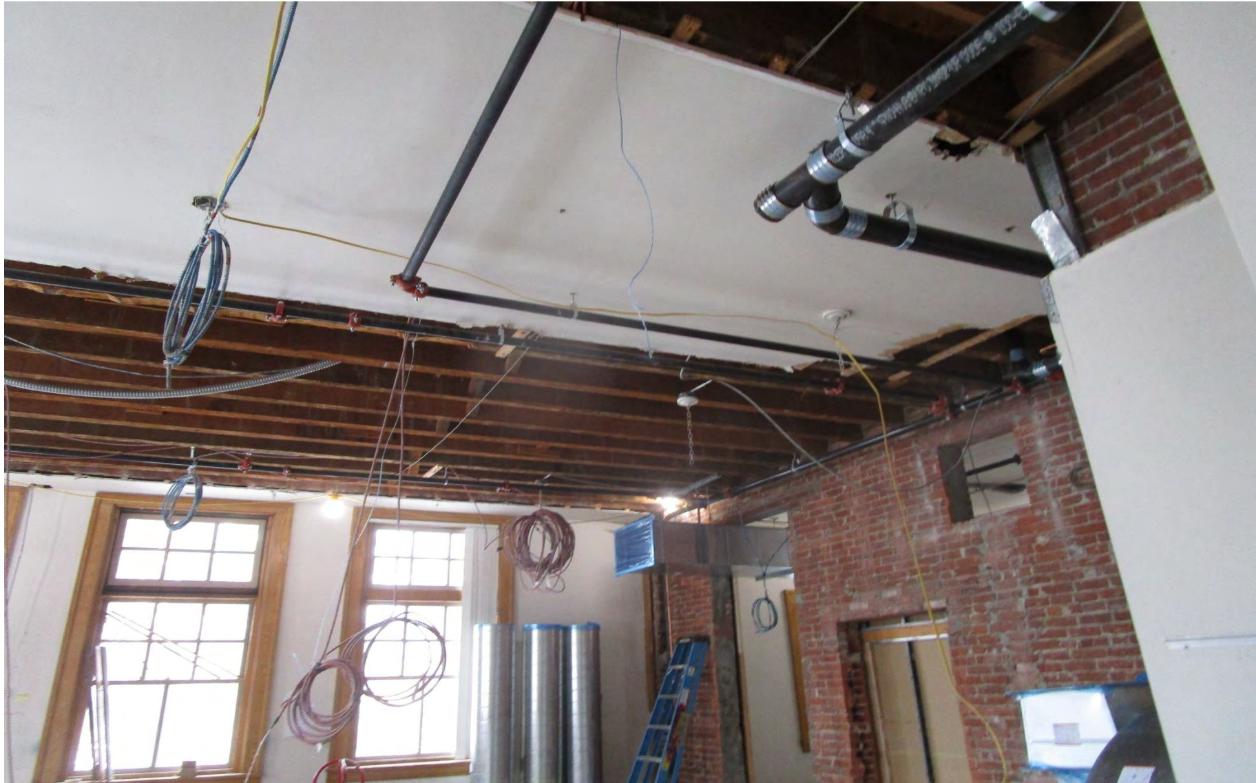
Kitchen ceiling area that requires additional LVL reinforcement framing
