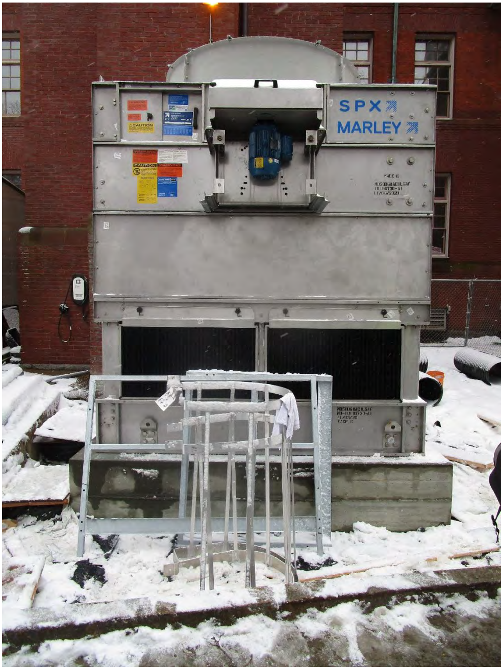
New cooling tower adjacent to north parking lot
