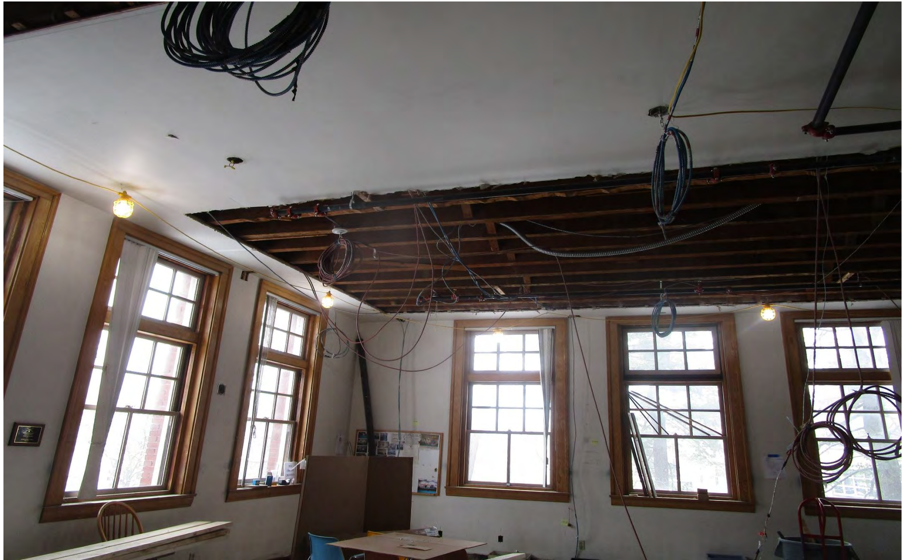
Kitchen ceiling area that requires additional LVL reinforcement framing
