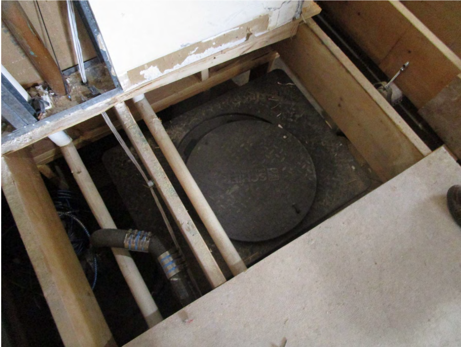
Grease trap for 1 st floor kitchen in Ground floor level crawl space
