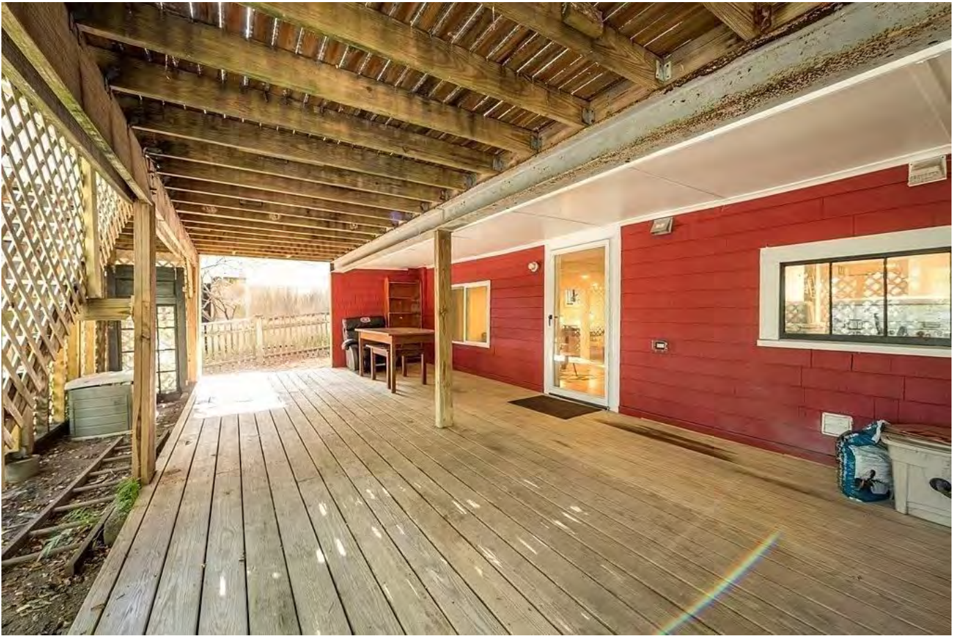
Underside of rear deck structure – to be reinforced and enclosed
