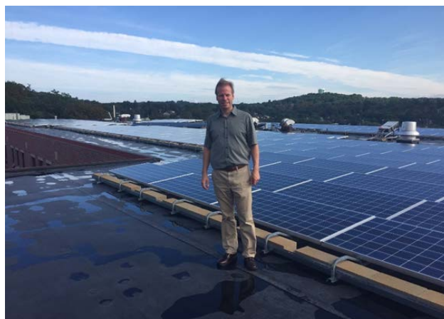
Solar array, Ottoson Middle School
