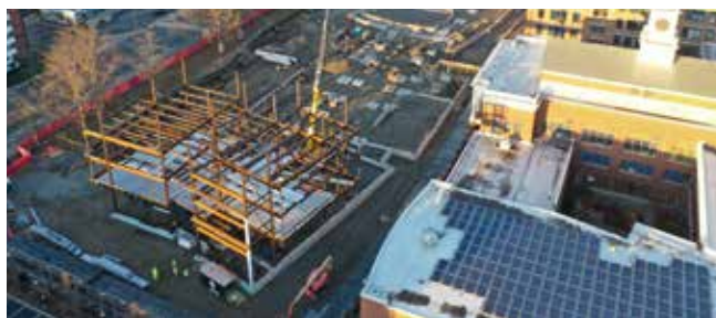
Construction of the new STEAM (Science, Technology, Engineering, Arts & Mathematics) classroom wing, December 2020
