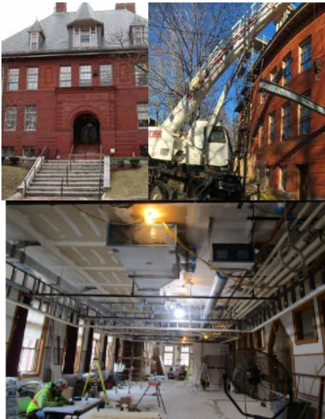
Central School / Arlington Community Center project. top left: west entrance, rigging in beam for first floor, and ductwork and ceiling installation on first floor.
