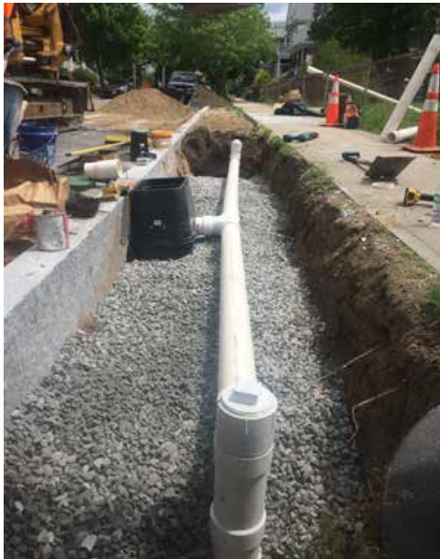
Infiltration trenches constructed in East Arlington connect to existing catch basins. Infiltration trenches collect stormwater runoff and remove pollutants before the stormwater enters the municipal stormwater system and travels to a water body, like Alewife Brook.
