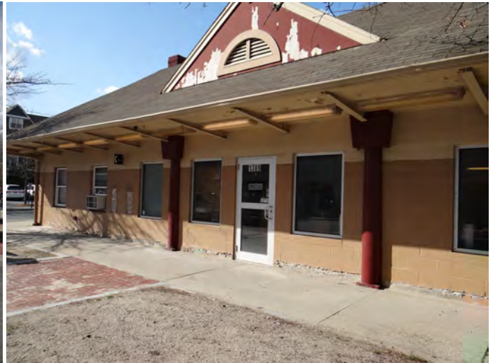
MBTA Bus Depot building with peeling paint, Arlington Heights. Photo: FinePoint Associates
