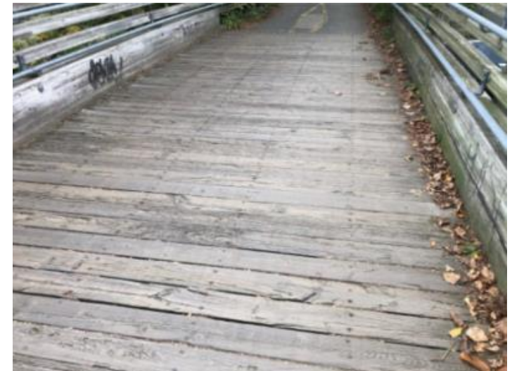
Bridge surface is worn
