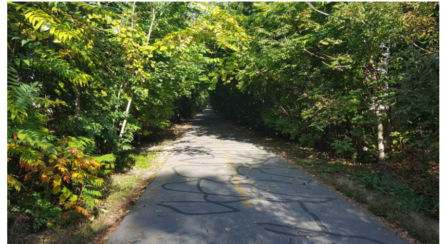
Crack sealing and overgrown vegetation
