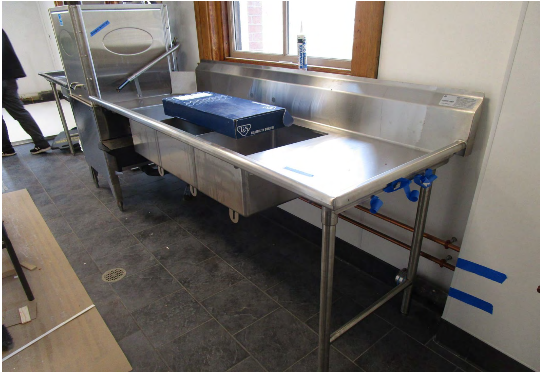
Dishwasher and sink in kitchen
