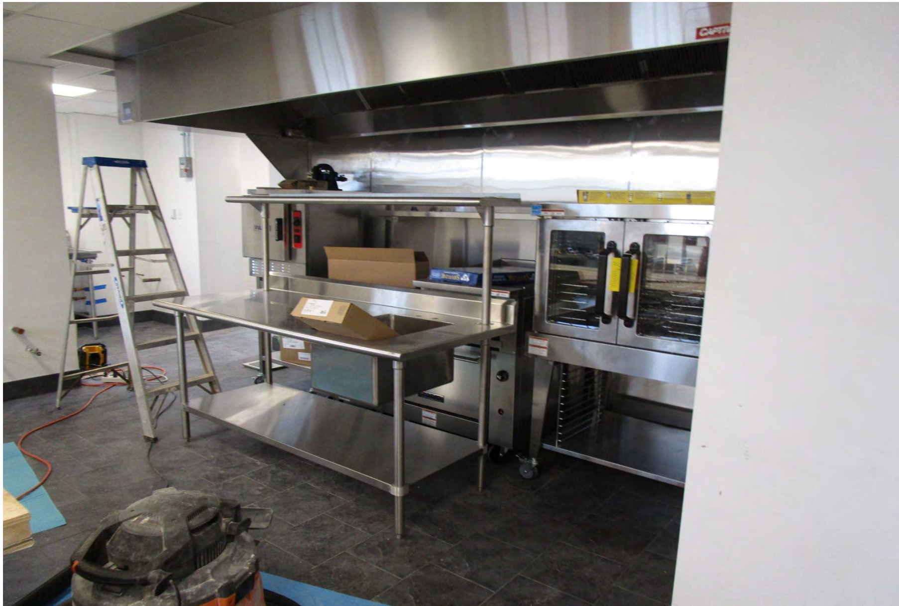
Stove and appliances installed under the kitchen hood
