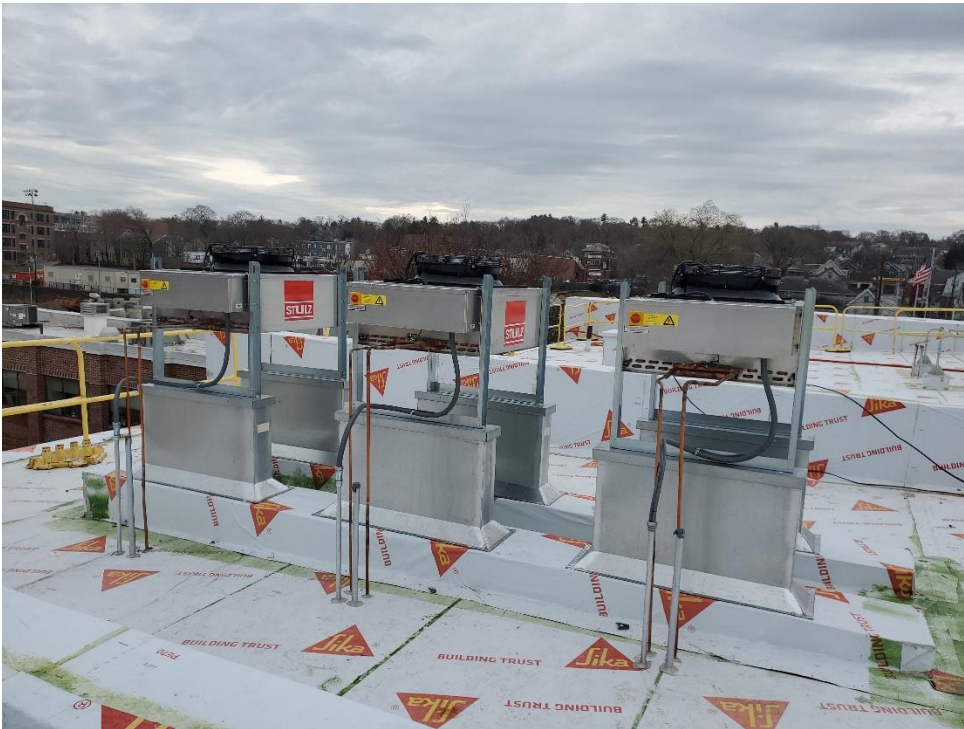
Photo # 1 – Rooftop Equipment (12/16/2021).
