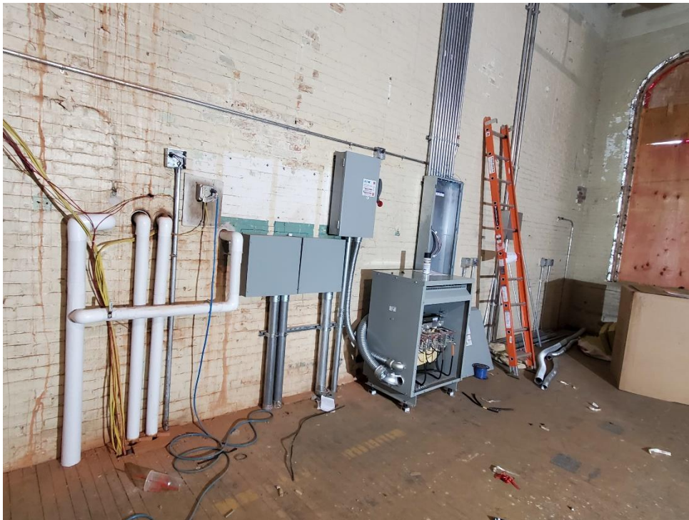
Photo # 2 – Electrical Equipment in Building A (12/15/2021).
