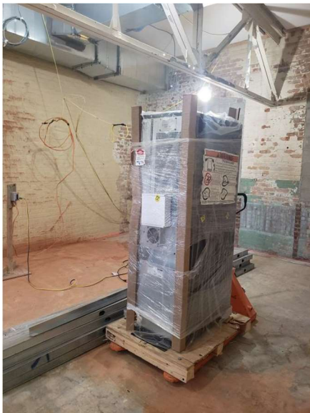
Future IS Server Room
