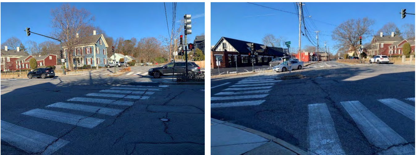
Figure 13 (Left) view looking north at cracked pavement within the crosswalk from the southeast corner of the Summer and Mill/Cutter Hill intersection. (Right) Looking west from wide turning radius and apex ramp to a small median.
