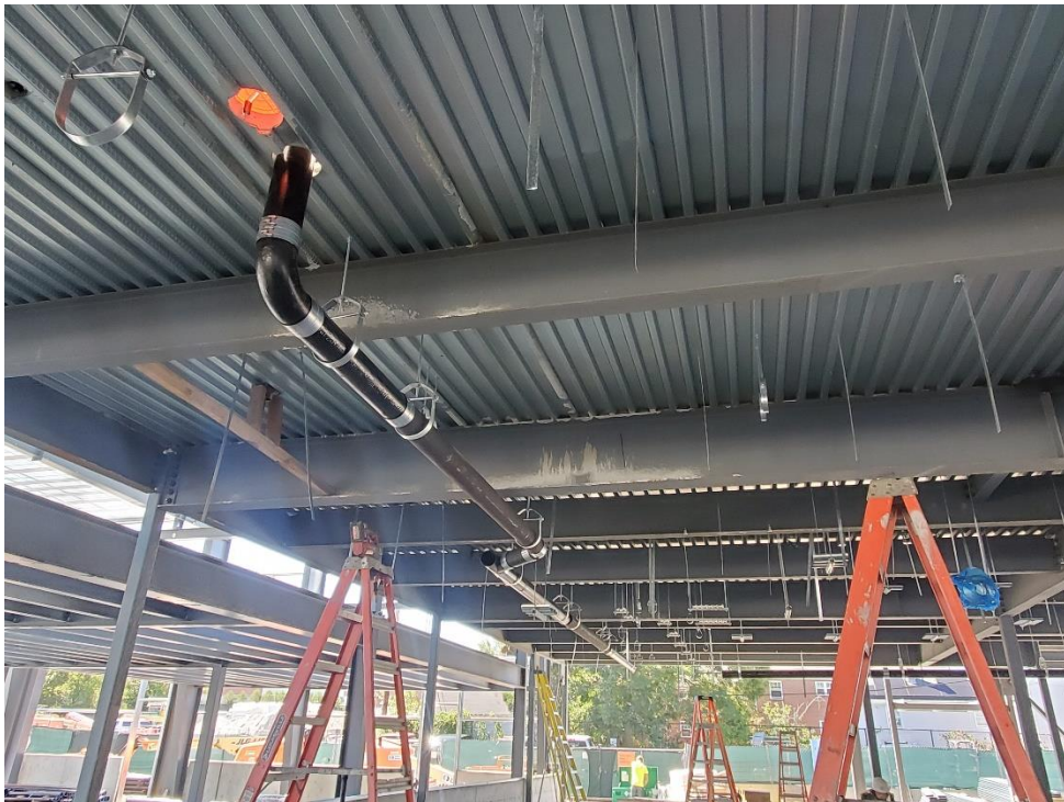
Photo # 2 – Domestic Water Lines & HVAC/Ductwork Hanger Installation at Building E 1 st floor (9/8/2022)
