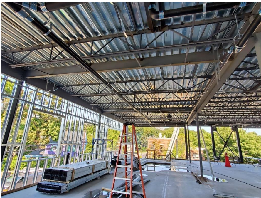
Photo # 4 – Domestic Water Lines, HVAC/Ductwork Hanger Installation and Cold Form Metal Framing at Building E 2 nd floor (9/8/2022)
