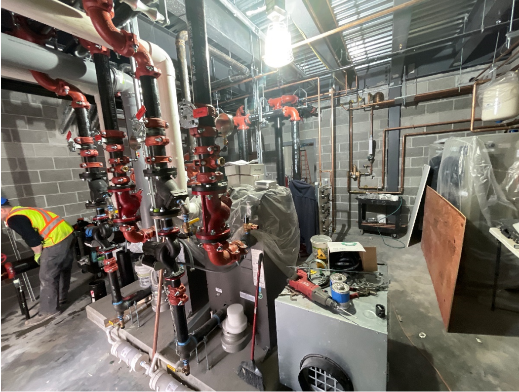
Photo #5 – Building E Maintenance Mech/Plumbing/FP Room (2/9/23)
