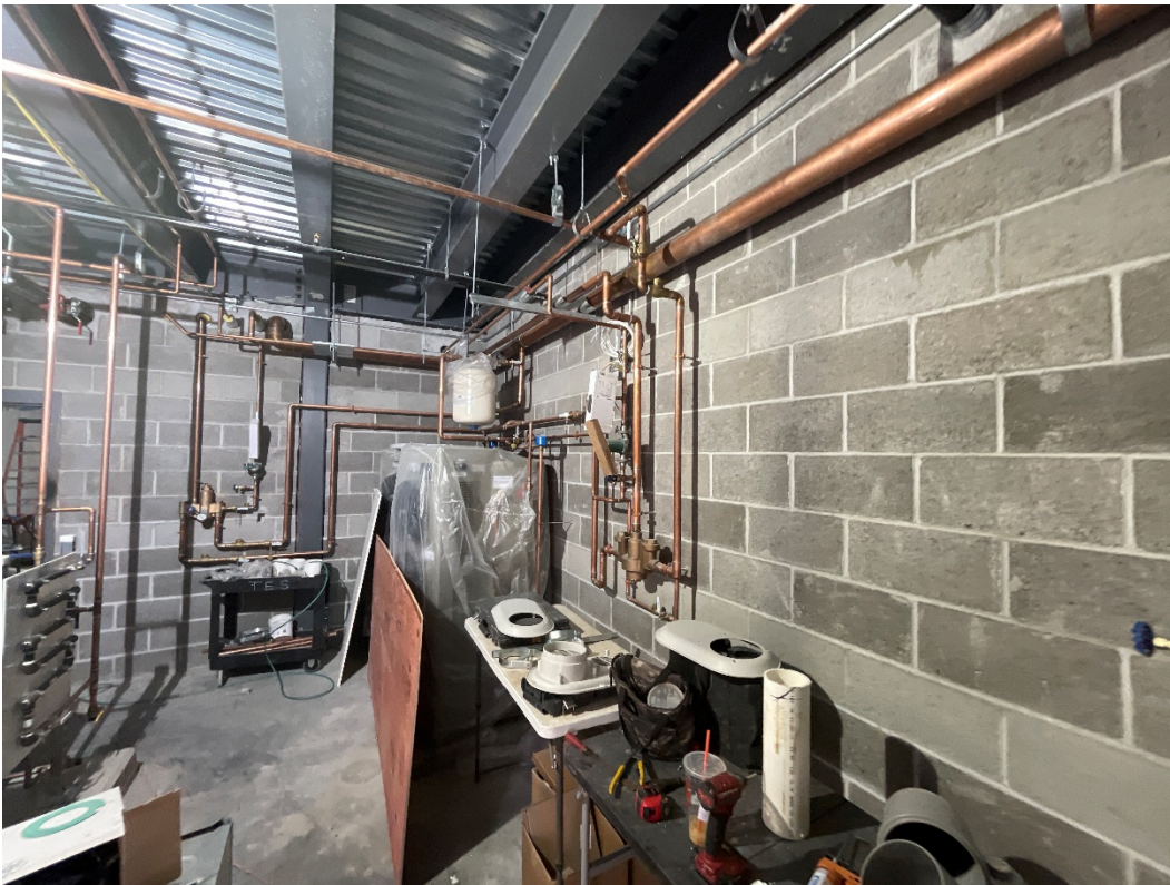
Photo #6 – Building E Maintenance Mech/Plumbing/FP Room (2/9/23)
