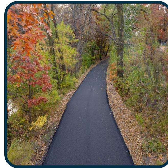
ADA Asphalt Path (along hillside with metal or granite edging, to match existing Robbins paths)
