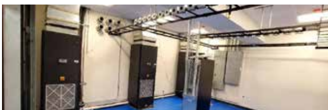
Building A IT server room – ready for server installation.
