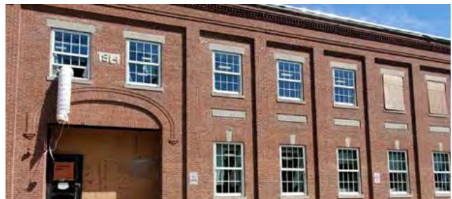
Building A exterior, showing new windows and disconnected cooling duct.
