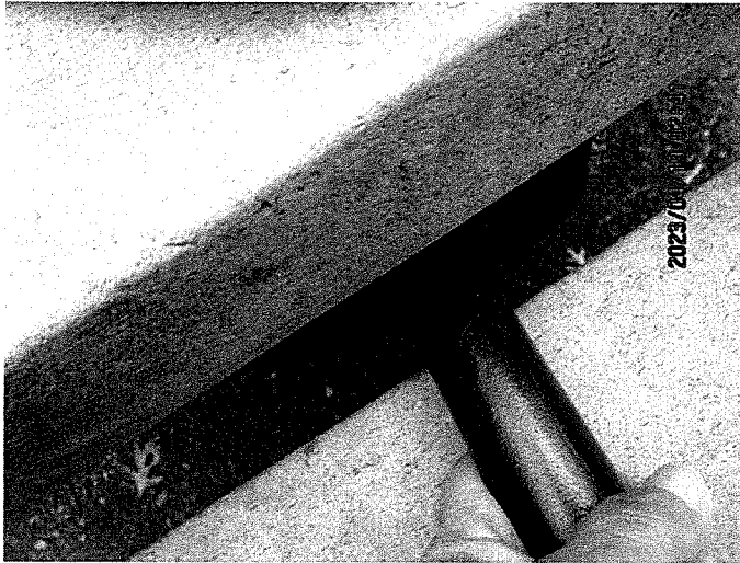
Head Entrapment deck/deck
