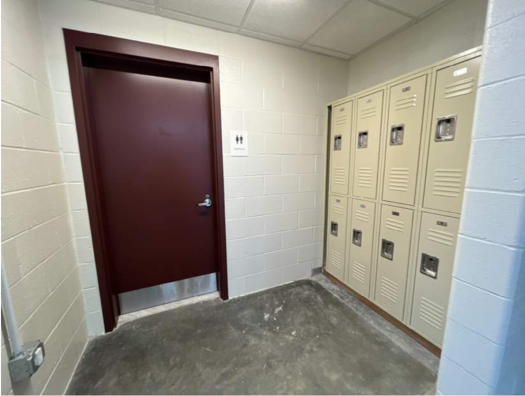
Photo #5 – Building E Maintenance Locker Alcove (6/12/23)
