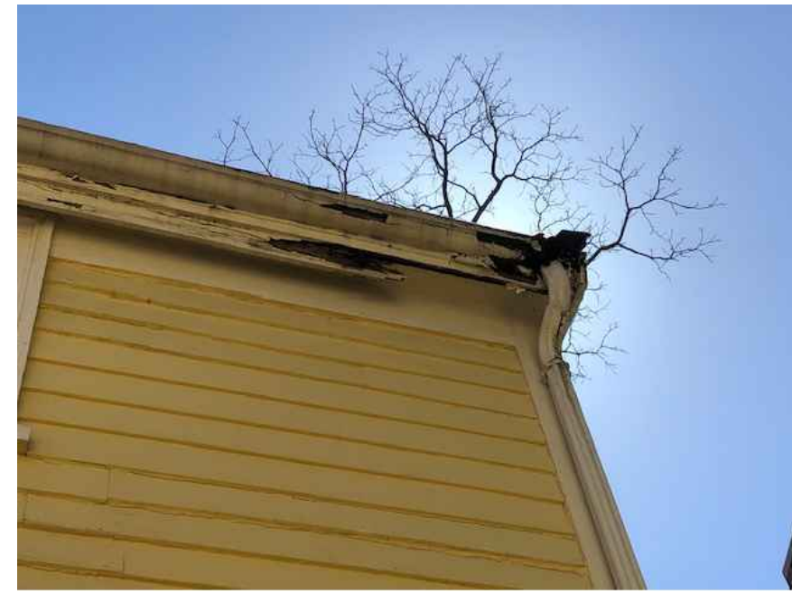
REMOVE & REPLACE ROTTING CORNERBOARD
