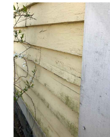
REMOVE, REPLACE, PRIME & PAINT CRACKED SIDING 4-1/4"x14-1/2" 4-1/4"x16-1/4"
