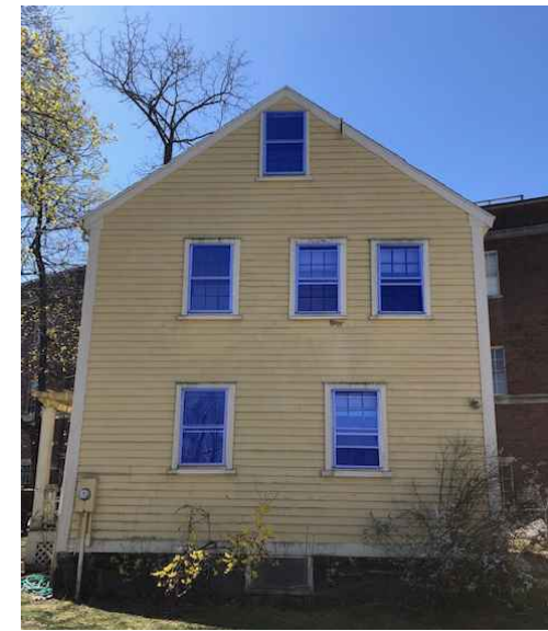
REMOVE & DISCARD STORM WINDOWS; SCRAPE CAULKING AND PATCH HOLES WITH PUTTY, TYP.
