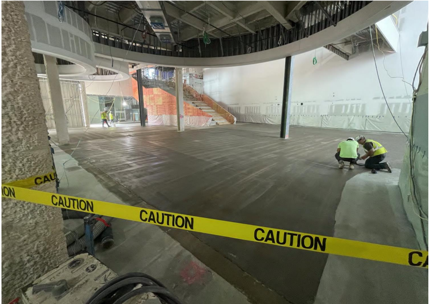
Photograph 4: Prepping the concrete slab for terrazzo flooring of the forum and cafeteria
