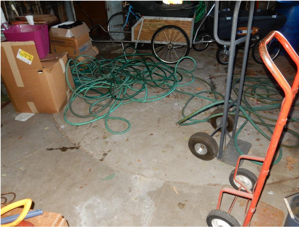
23. Remnant of former car turntable. Surrounding concrete floor appears original. Circular infill concrete appears tight to surrounding concrete, more recent, and not operable.
