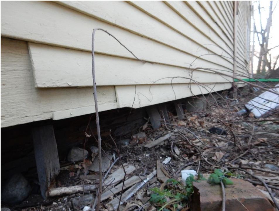
8. Missing sections of clapboard siding and course of cinder block foundation.
