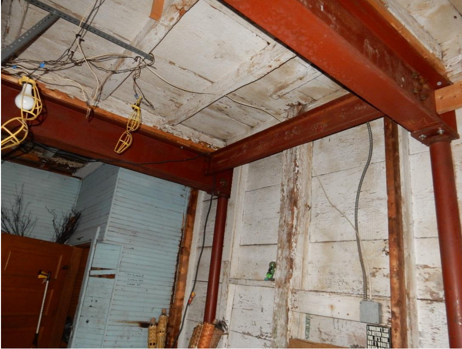
19. Underside of second floor framing in two-story building. Steel beams are supported on pipe columns in wall next to one-story building.
