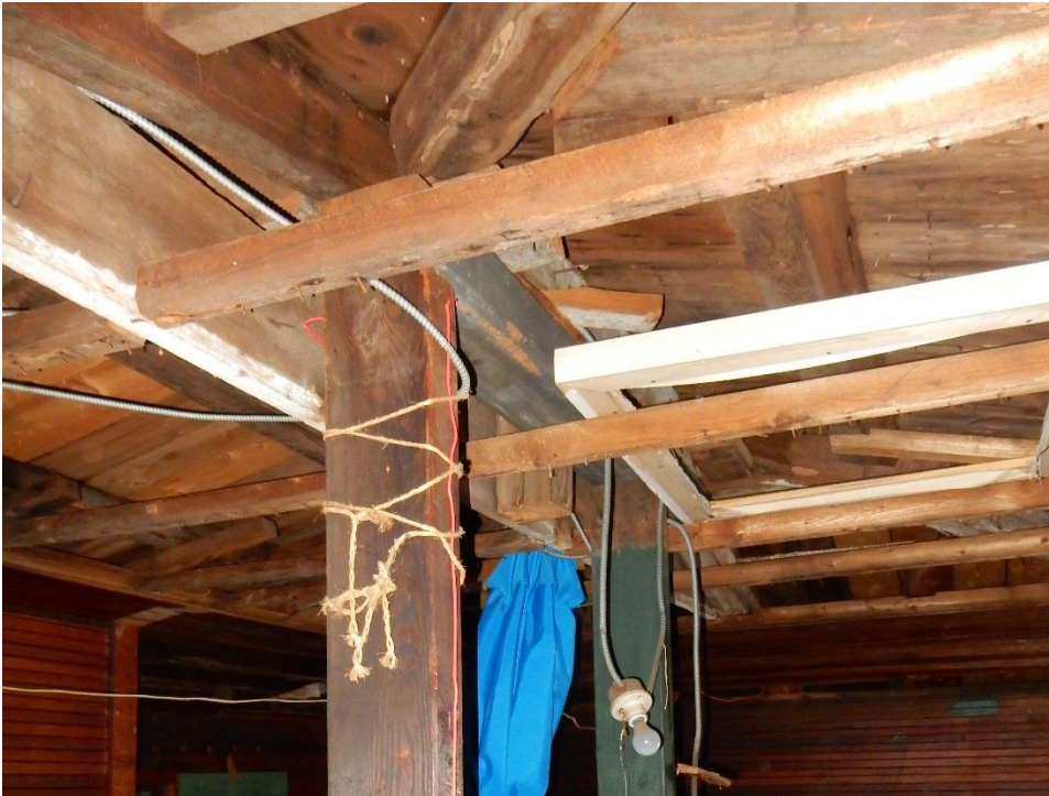
22. Two wood shoring posts support the ends of a 5x5 ridge beam. Ridge beam has a 2x10 lapped and nailed to the sloping 5x5 rafters that align with the ridge beam. This formed a makeshift truss and was the main support for the roof.
