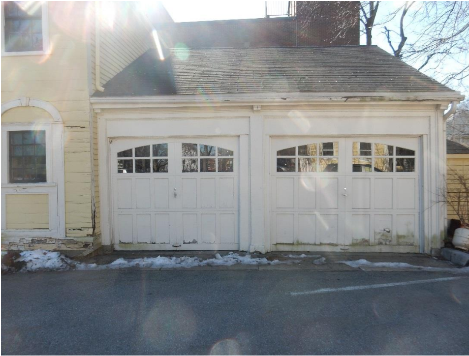
7. At north face of one-story area, rot is present in gutter, corner trim of two-story section, and bottom trim and panels of doors.
