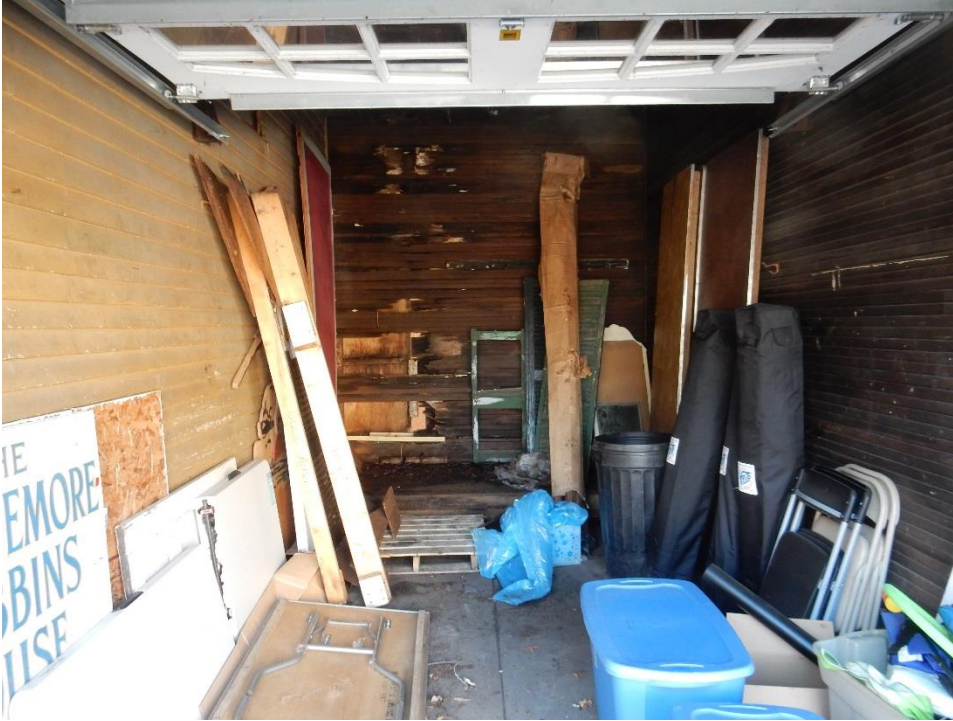
11. Bay in one-story portion next to two -story area. Rear bead board facing is heavily rotted. Some evidence of mold is present in the bead board on the wall separating the west most bay. Raised platform in background is covered with rotted debris.
