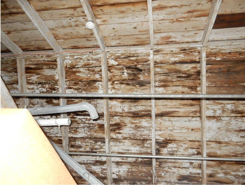
15. Roof framing over aforementioned bay. Rafters appear intact. Board sheathing has dark staining (potential mold/rot) from past moisture.
