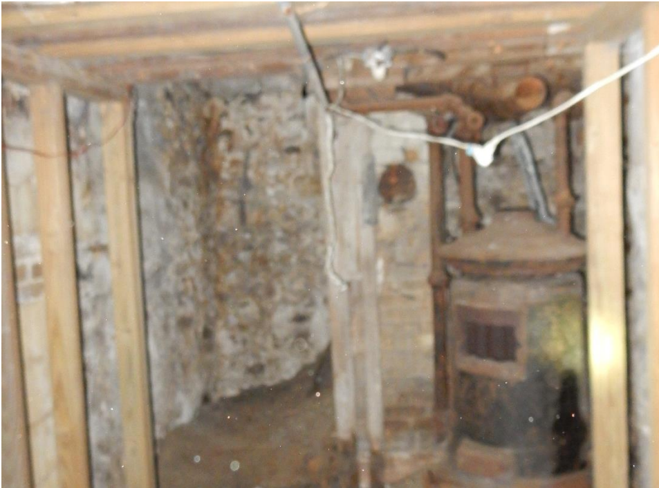
10. View within basement that fits under a small portion of the first floor. Wood studs along two sides support closely spaced planks to shore the concrete slab. Chimney and abandoned boiler in background.
