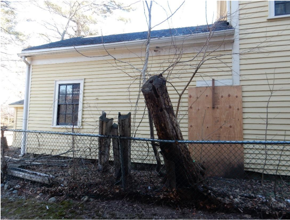
5. West end of South face of Whittemore Robbins Carriage House. Plywood panel propped against a rotted hole in the wall. Note: lintel trim is present that suggests a former wall opening.
