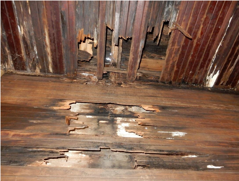
12. Soffit bead board in the aforementioned bay is rotted near the rear wall.
