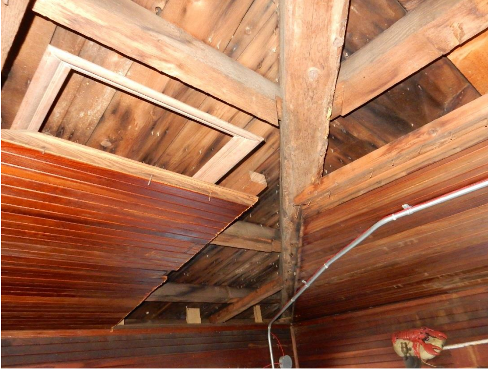
21. Underside of two-story building roof. 3x4 purlins are supported on 5x5 hip beams. Ceiling and walls originally covered with bead board.
