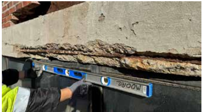
Deteriorating lintels to be repaired or replaced on Building D.
