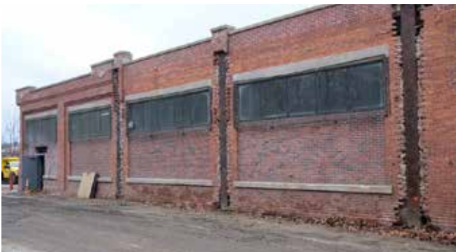
Exposed columns to be repaired and filled on Building D.
