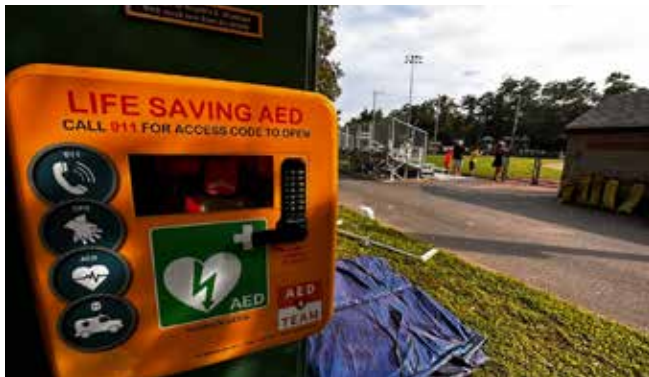
AED installed at Buck Field/Hills Hill Field on Summer St.
