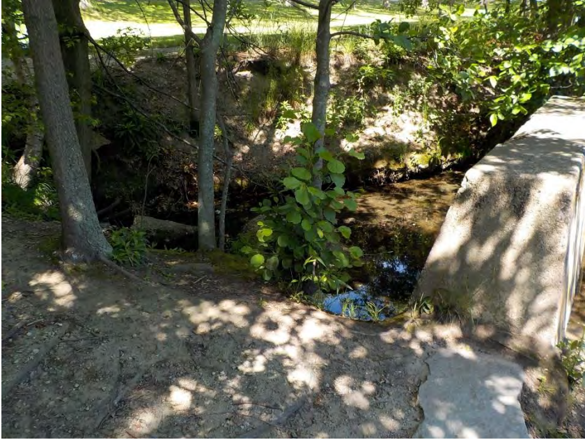
Photo #5: South side of Mystic River, Mystic River Parkway between Location #1 and River Street. Pipes discharge to river, and in a number of locations, contribute to riverbank erosion. (Location #3) (Photo Taken: 06/10/16)
