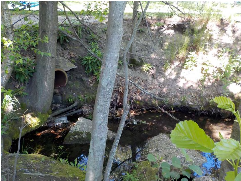
Photo #6: South side of Mystic River, Mystic River Parkway between Location #1 and River Street. Pipes discharge to river, and in a number of locations, contribute to riverbank erosion. (Location #3) (Photo Taken: 06/10/16)
