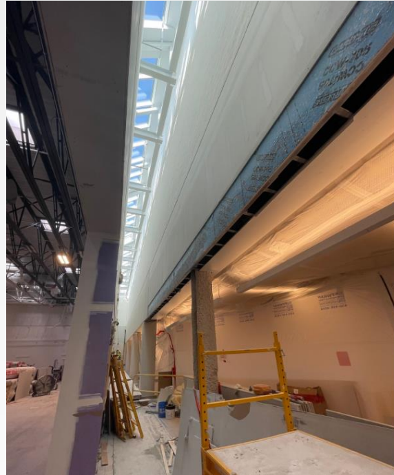
PH 2 + 3 Tie In Point
